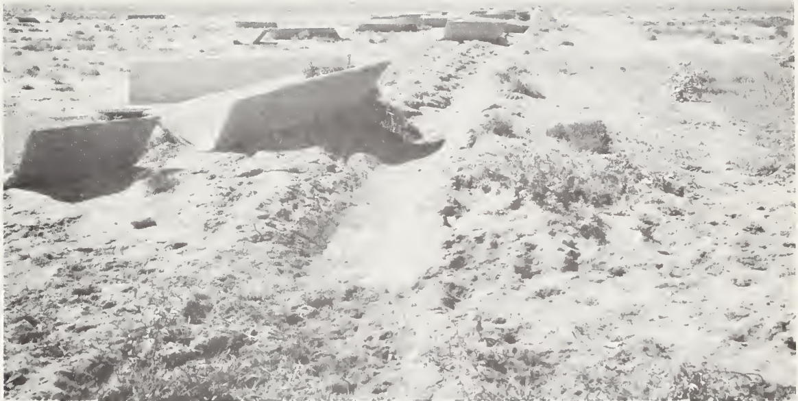
Floodwater damage from flood of August 1966 to irrigation systems in the Wild Horse farming area.
