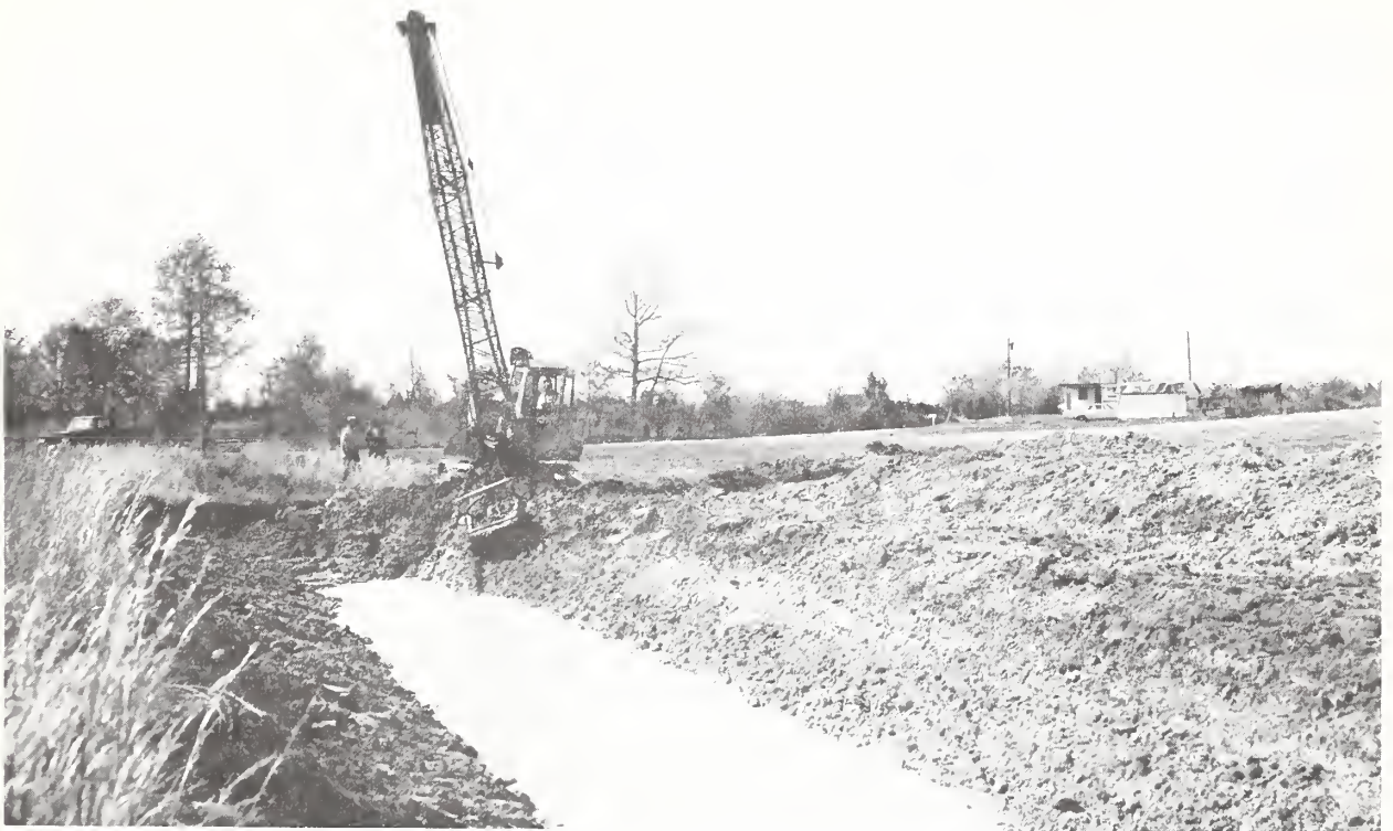
RECONSTRUCTION OF DITCH SIMILAR TO ABOVE CONDITIONS. NOTE WORK FROM ONE SIDE -- SPOIL DUMP IS BACK FROM DITCH TO ALLOW ACCESS ROAD FOR MAINTENANCE.
