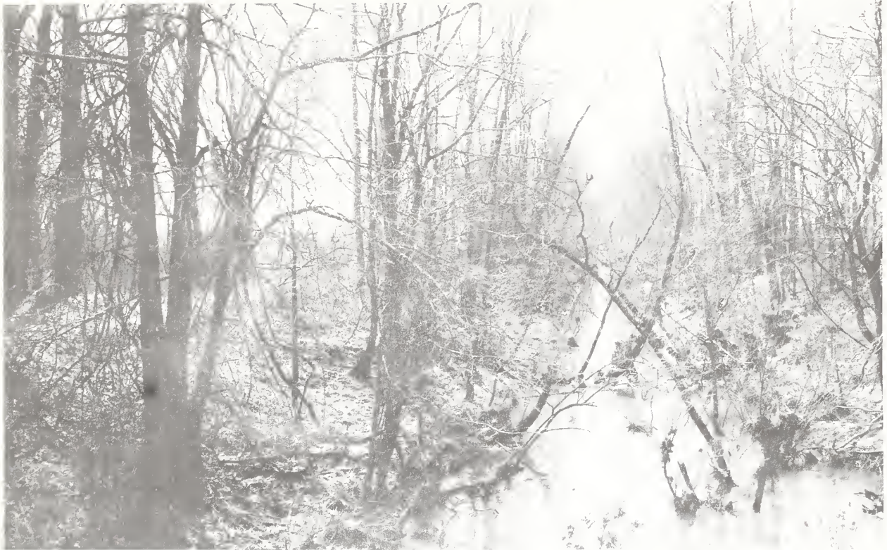
THIS PICTURE SHOWS THE CONDITION OF THE DRAINAGE DITCHES WHICH SERVE AS OUTLETS FOR LATERAL DITCHES AND ON-FARM DITCHES. RENOVATING OF THESE DITCHES BY THE PROJECT WILL IMPROVE DRAINAGE AND REDUCE FLOODING. CONSTRUCTION WILL BE FROM ONE SIDE TO PRESERVE TREES AND BRUSHY COVER ON THE OPPOSITE BANK FOR WILDLIFE HABITAT.
