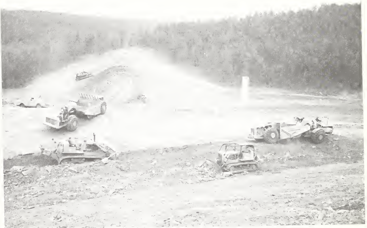
CONSTRUCTION SCENE DURING CONSTRUCTION OF FLOODWATER RETARDING STRUCTURE. NOTE INLET RISER ON UPLAND SIDE.
