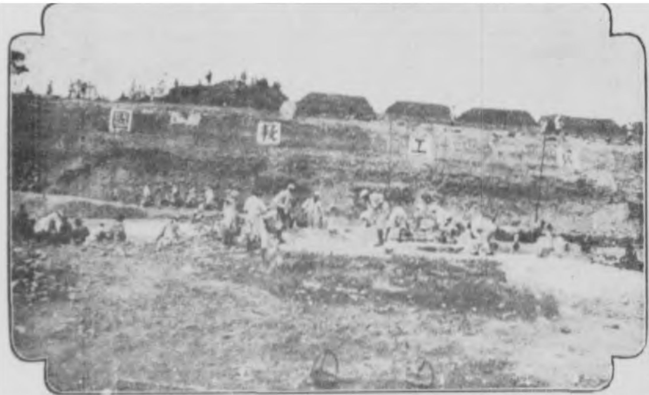
Gen Feng's soldiers busy at digging earth for building the dams of Yung Ting River (The four Chinese characters on the wall meaning "Saving China by Soldier-laborers")
