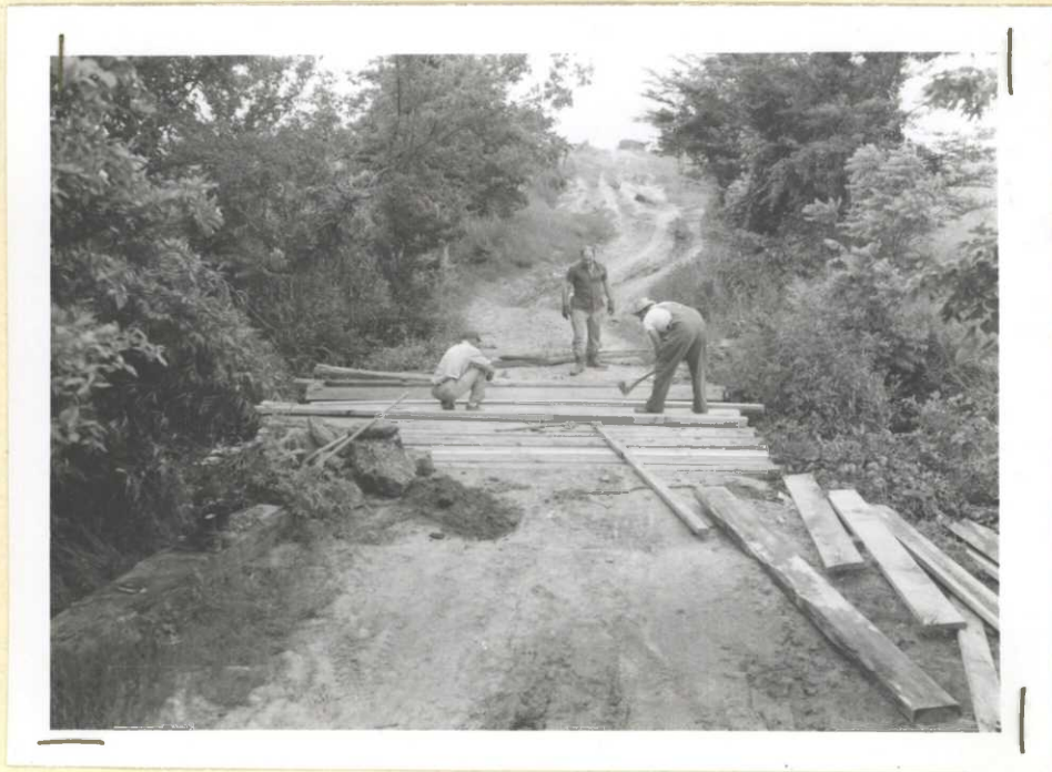
Personnel rebuilding truck trail bridge at Sulphur Wells Area, Big Sandy Refuge Area., May, 1950.
