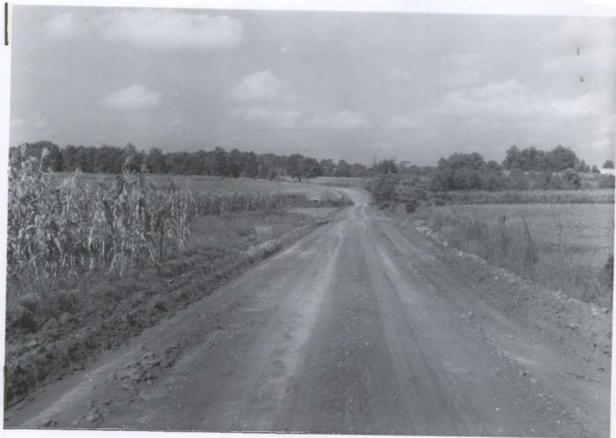
After shot, October 1950, showing new road and drainage, and waterfowl crops at Sulphur Wells. Soil and Moisture Operation.
