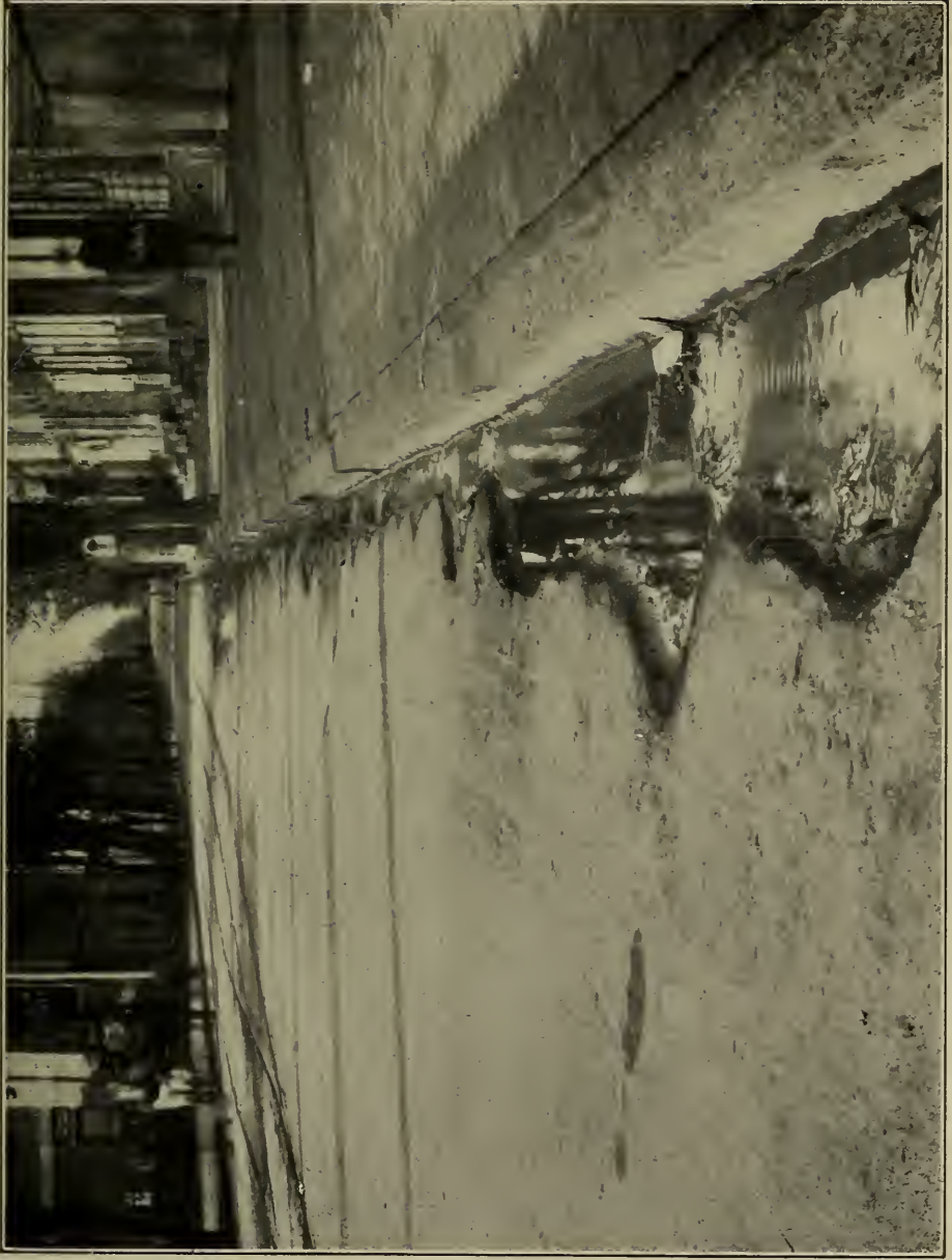
FIG. 27.—Bermudez Asphalt Surface Disintegrated by Water.
