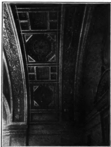
Ceiling treatment adapted from the Villa Madama which adds richness in color and gives broken surface to hinder echoes. Greenwich, Conn.
