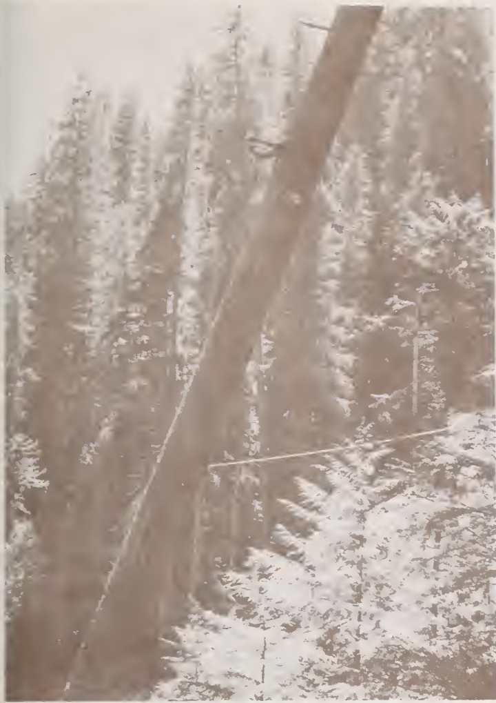
Figure 18. Cable-assisted felling keeps trees out of stream channels and it also reduces breakage of the trees since they are felled uphill. Less residue results and damage to streams is reduced. Oregon State University, 870
