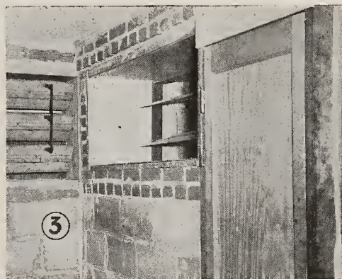
Plenum or air mixing chamber.
