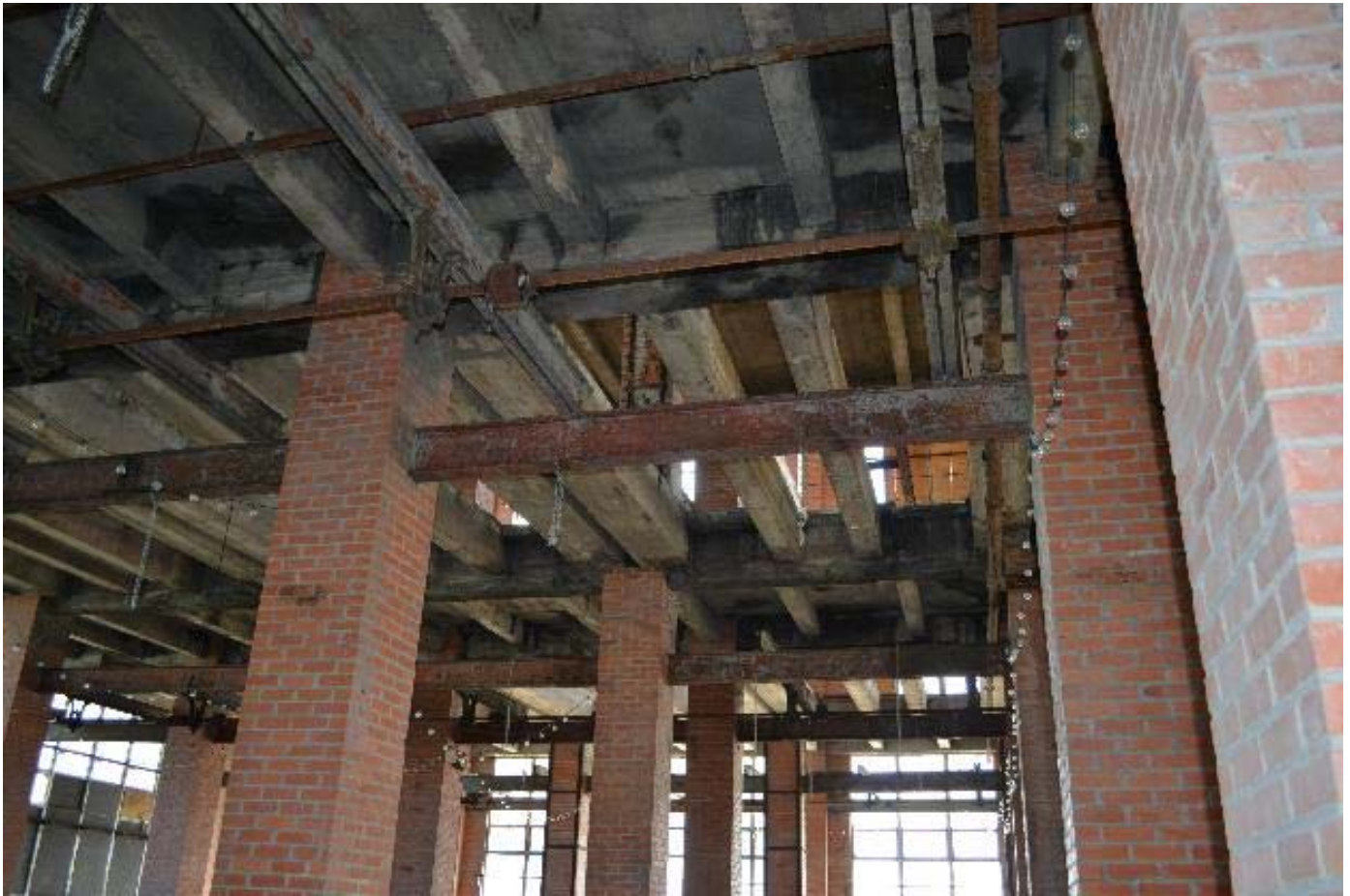
Photo 21 - Char House (Resource ID 1), interior, missing flooring visible, view south
