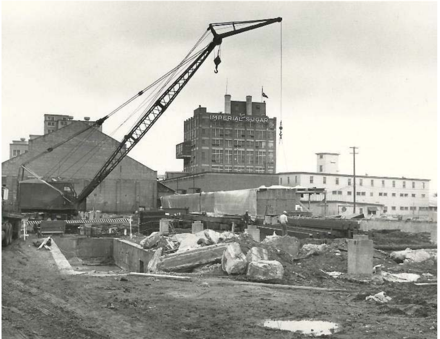
Figure 10 - During construction of a new warehouse, c. 1969. Courtesy Sugar Land Heritage Foundation.
