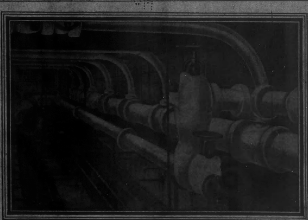
CRANE PIPE BENDS RELIEVE EXPANSION STRAINS IN THIS NORTHWEST PAPER CO. PLANT. G. F. HARDY, ENGINEER
