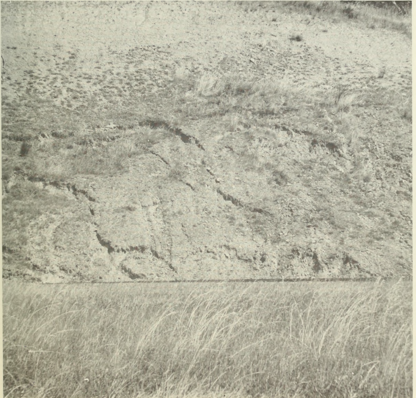
Figure 29 Slope failure and resultant severe rill erosion along road cutbank slope in Etelka (557) and Whobrey (501) soils of Otter Point Formation.
