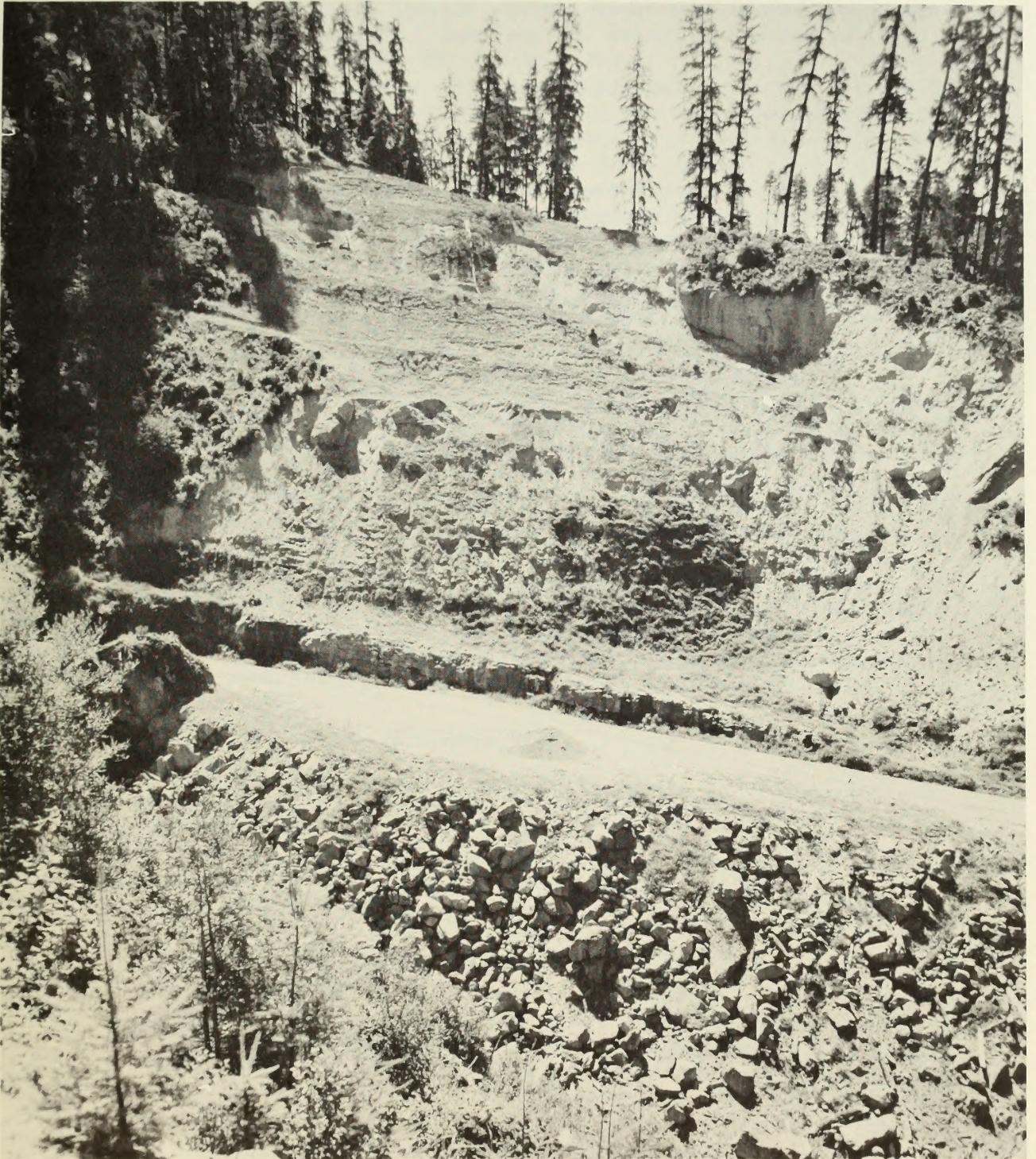
Figure 10. Major Slide Correction in cutbank slope of access road located in the Elkton Formation. Visible slumps occurred subsequent to correction.
