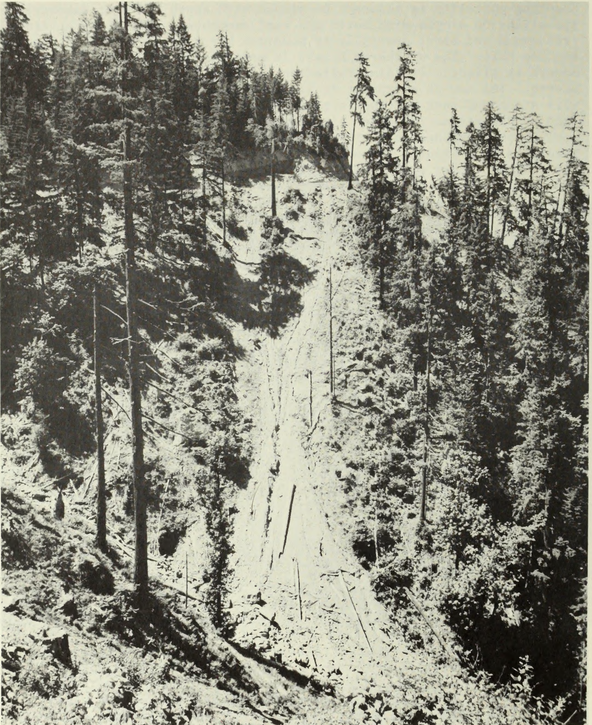
Figure 22 Loss of site productivity from debris avalanche type of slide due to sidecast of waste materials during road construction.
