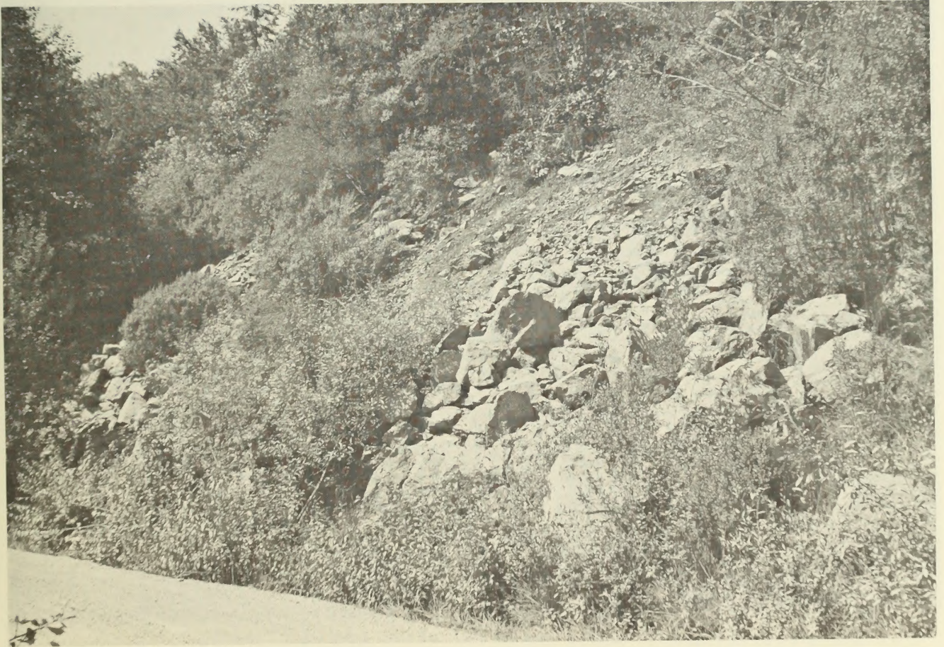
Figure 31 Rock ballast placed along the toe of cutbank slope for stabilization of road cutbank in the Otter Point Formation.
