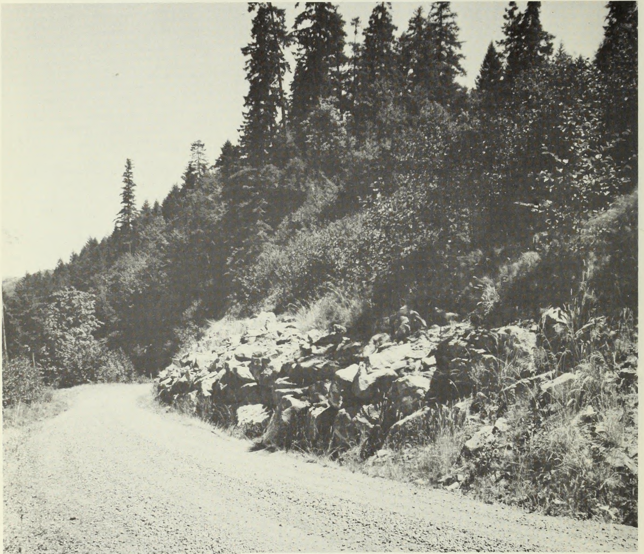
Figure 9. Rock Buttress at toe of slope in slide correction. Elkton Formation in Type II Terrain along Heddin Creek BLM road.
