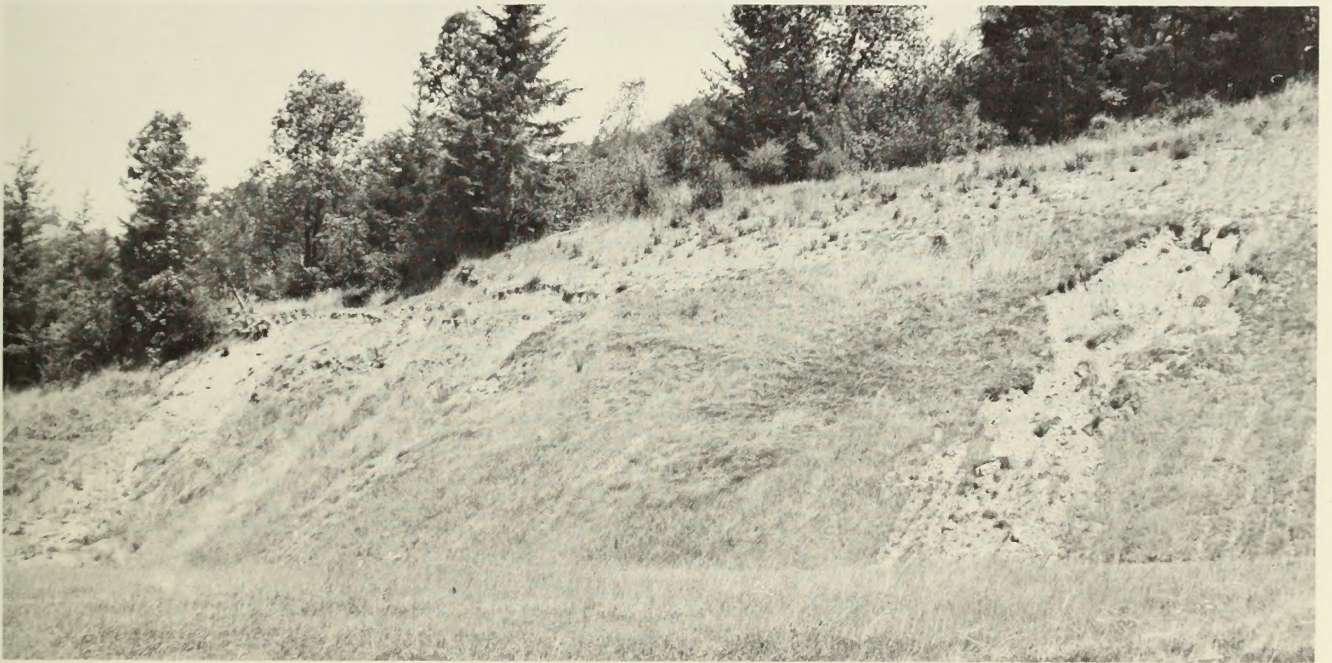
Figure 27 Cutbank slope failures in one year old established seeding due to piping on Whobrey (501) and Etelka (557) soils of the Otter Point Formation. Sources of pore water pressure and seepage force are numerous seeps and flowing springs that outcrop along sideslopes.
