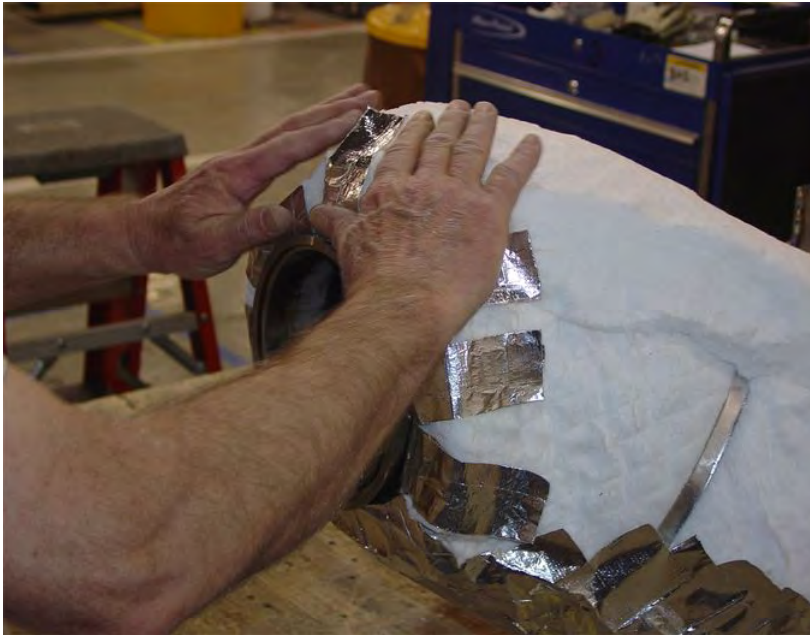
Figure 32. Attaching Top Piece of Insulation to the Rest of the Insulation (Sheet 1 of 2).
