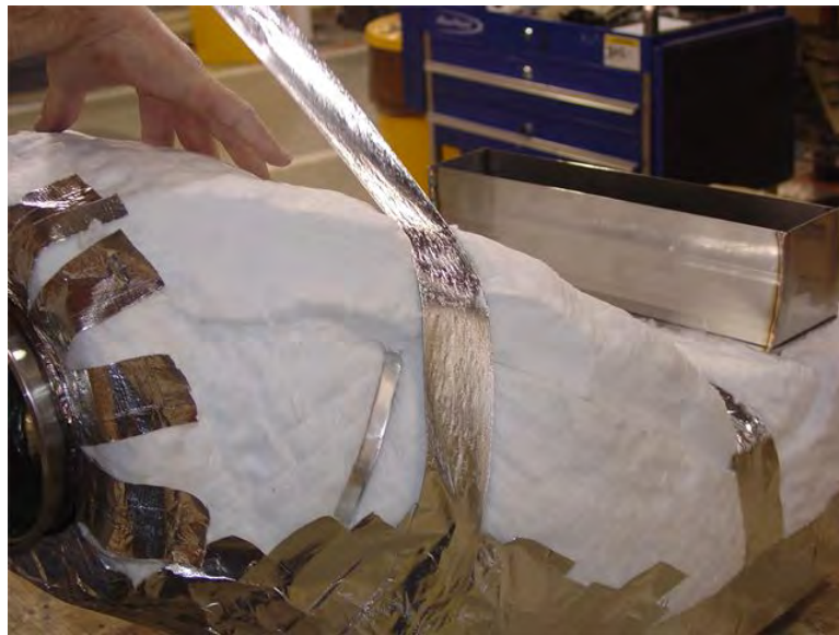
Figure 32. Attaching Top Piece of Insulation to the Rest of the Insulation (Sheet 2 of 2).
