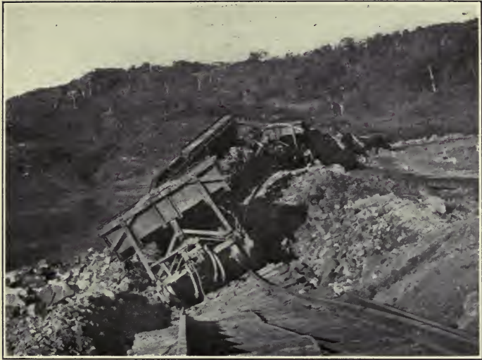
FIG. 14.—SLIDES INTO WET FILL, GATUN DAM.
