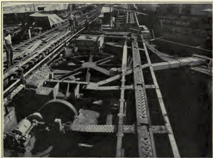
FIG. 21.—GATUN UPPER LOCKS, MITER GATE-MOVING MACHINE; STRUCTURAL STEEL GIRDERS FOR TOWING-LOCOMOTIVE TRACK SUPPORTS IN FOREGROUND. JUNE, 1912.
