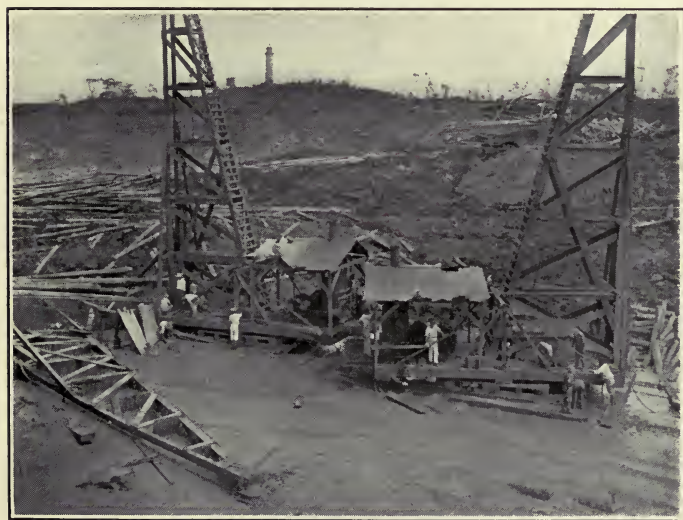
FIG. 9.—SLIDE INTO SPACE EXCAVATED FOR NORTH GUIDE WALL, GATUN LOCKS.
