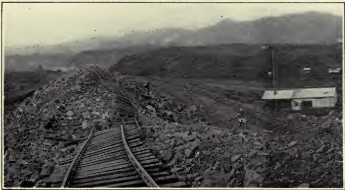
FIG. 13.—SLIPPING OF THE SOUTH TOE OF GATUN DAM, TOP VIEW, November 21, 1908.
