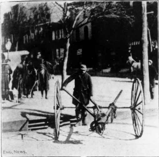
Fig. 3.—TRIPOD AND LIFT READY TO MOVE. APPARATUS FOR CLEANING SEWER CATCH-BASINS AT WILMINGTON, DEL.
