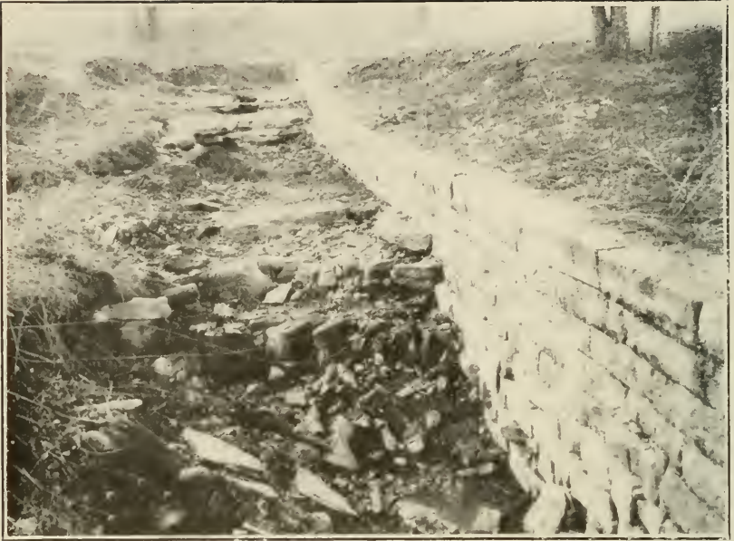
Fig. 5. Spillway of the upper pond of Bloomington water-works, showing joints in the rock.
