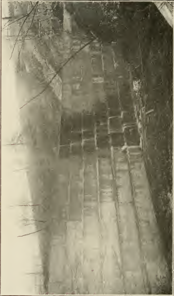
Fig. 2. Indiana University dam, seen from the valley below the dam. Each ledge is 4 feet high. Three ledges are concealed beneath the ground.
