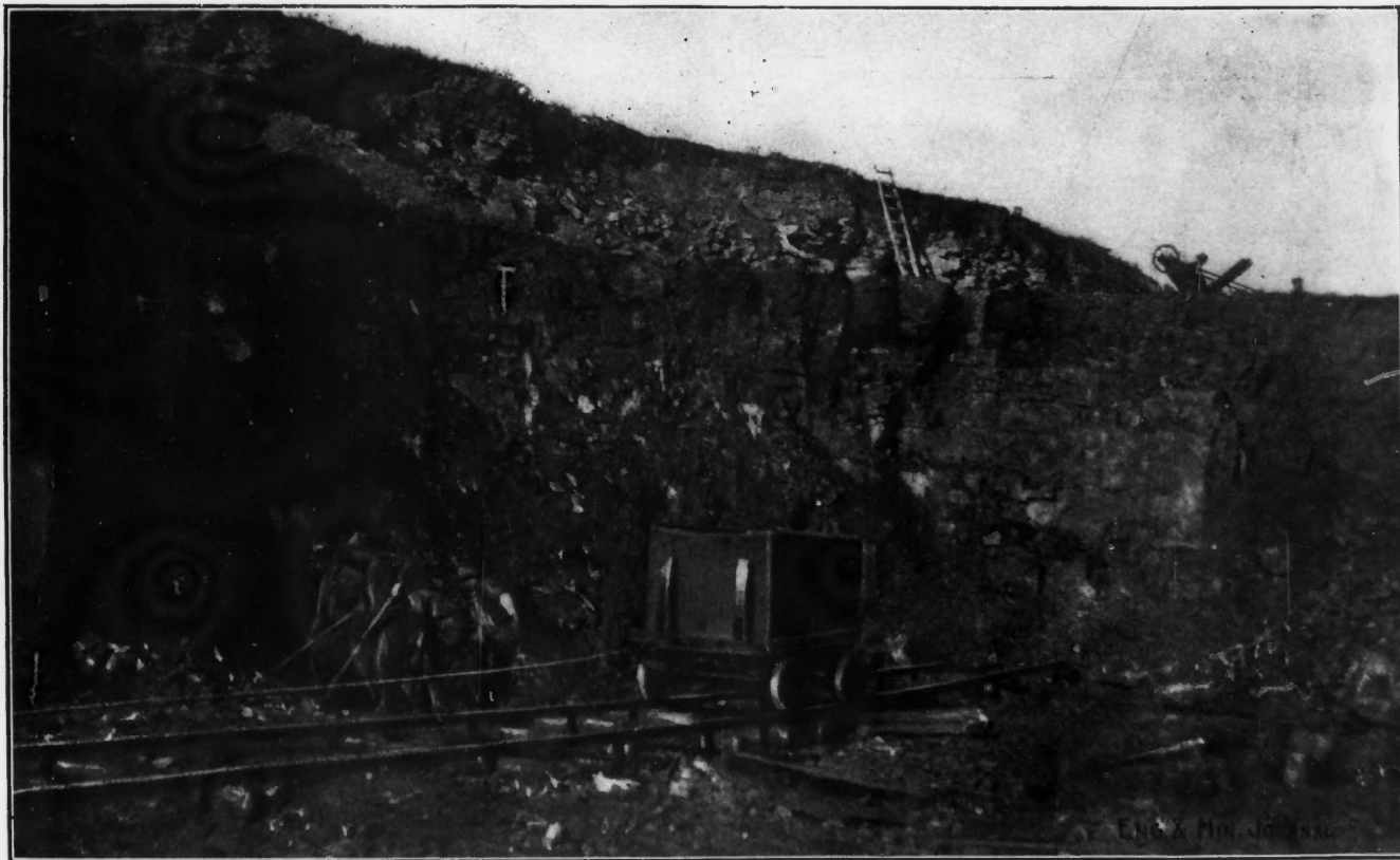
LOADING ORE DIRECTLY INTO SKIPS AT THE NORTH SIDE OF WASP NO. 2 OPENCUT; THE OVERBURDEN IS REMOVED BY STEAM SHOVEL
