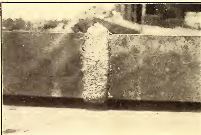
WELD AT BASE OF RAIL
