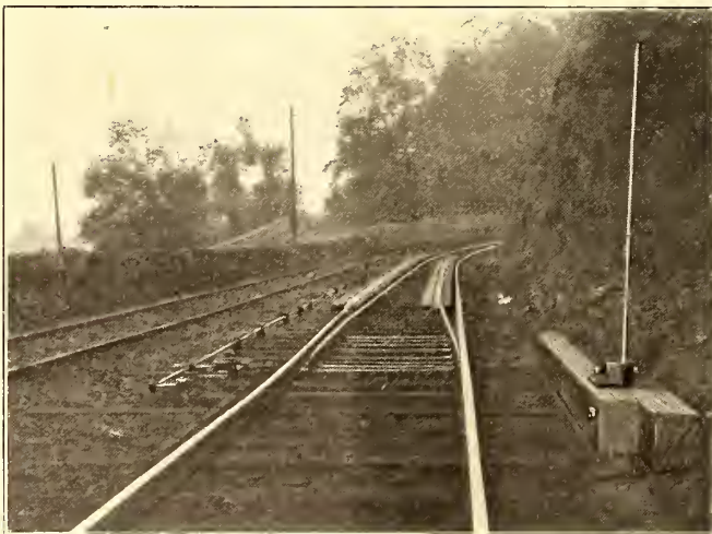
ENTRANCE TO SANDED TRACK FOR STOPPING RUN-AWAY CARS—NEW JERSEY & HUDSON RIVER RAILWAY
