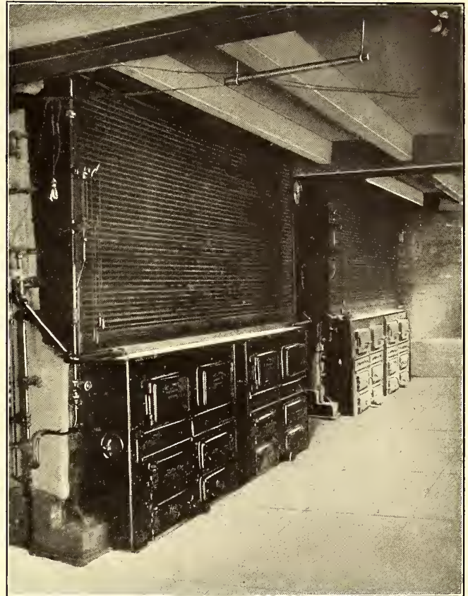
TWO OF THE 500-HP BOILERS IN THE BASEMENT
