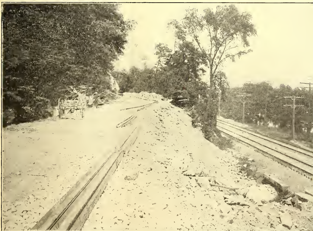
FILL BETWEEN EAST LIVERPOOL AND WELLSVILLE
