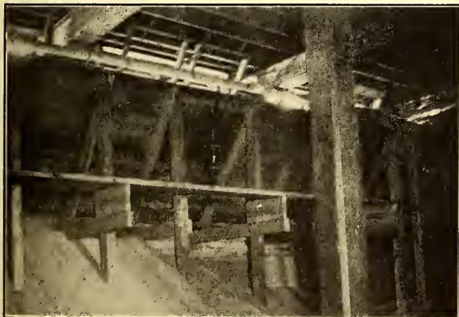
SAND DRIER EMPLOYING STEAM PIPES
