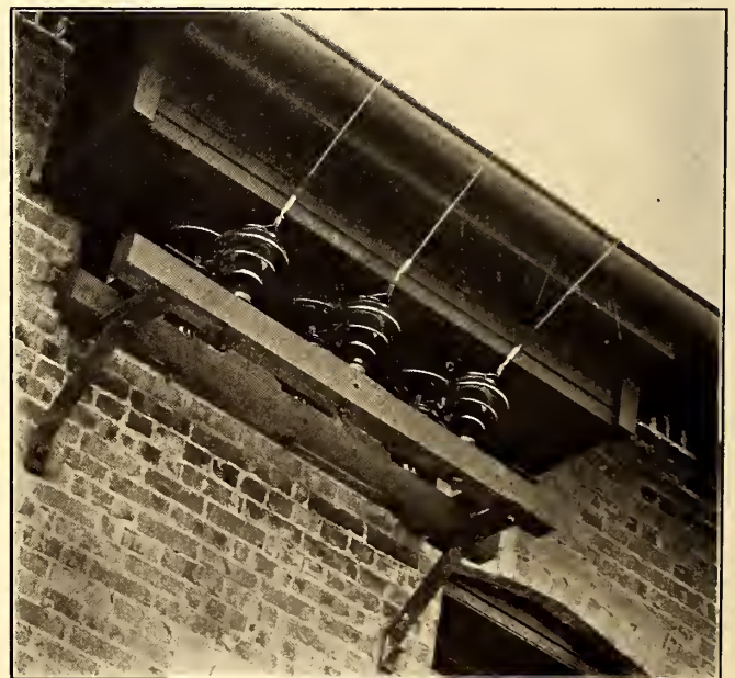
HIGH-TENSION WIRES ENTERING HERROLL SUB-STATION
