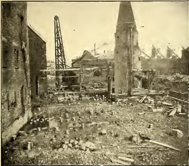
VIEW SHOWING THE PILING FOR THE SOUTH HALF OF THE PLANT, AND THE PORCUPINE BOILER SUPPLYING STEAM TO ENGINES IN THE BUILDING WHICH OCCUPIED THE SITE OF THE NORTH HALF OF THE PLANT
