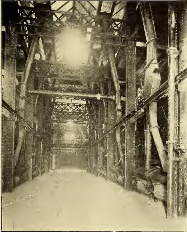
BOILER ROOM OF THE GREENWICH GENERATING PLANT
