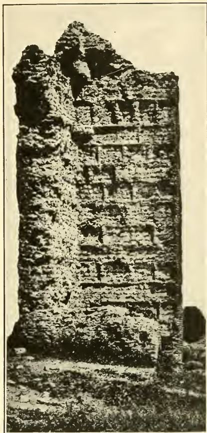
FIG. 1.—ONE OF THE PIERS OF THE AQUEDUCT OF CLAUDIUS, SHOWING THE COURSES IN ROMAN CONCRETE.
