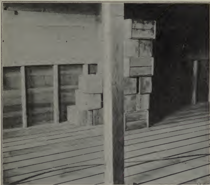
Fig. 7. Basement of Dr. Whitney's Wenatchee Valley storage, showing floor and wall construction.
