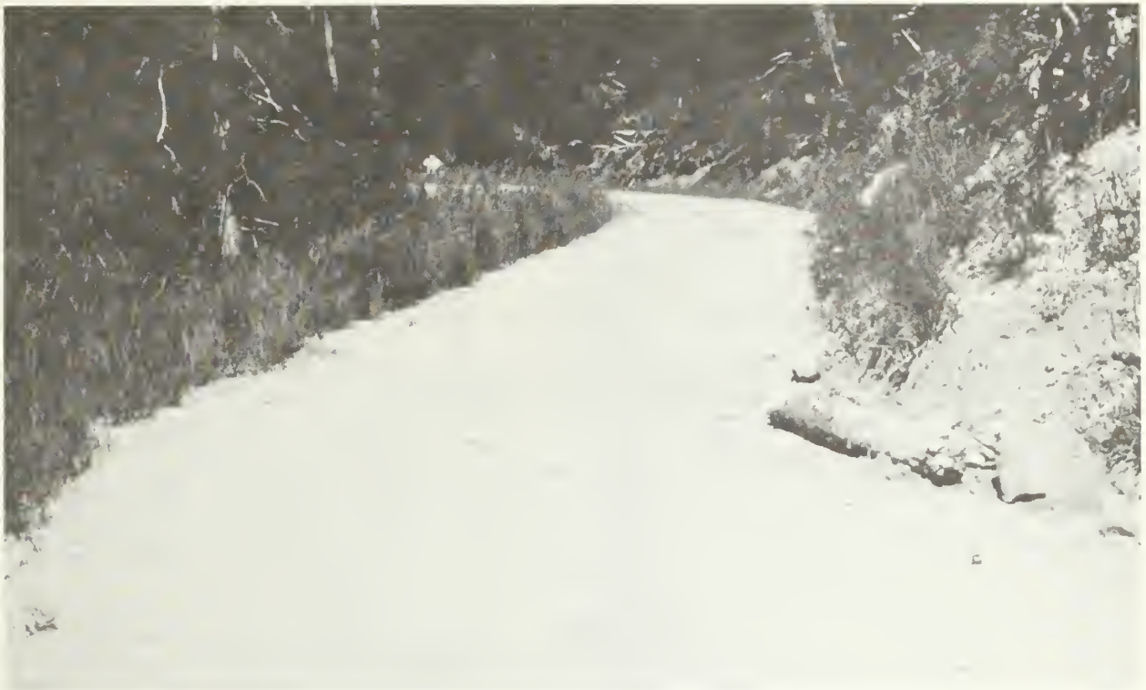
Figure 13.--Transition from outslope to inslope just past the curve is an example of good design functioning well.
