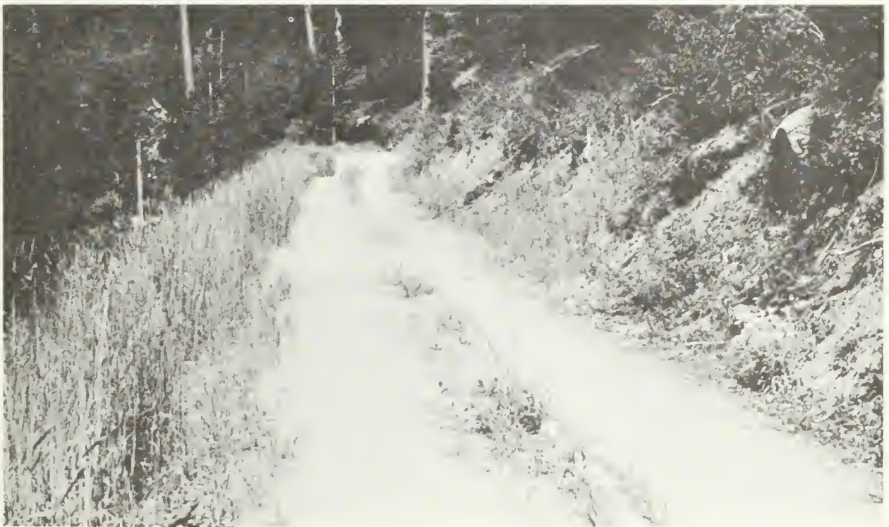
Figure 14.--Dip near the end of a section of outsloped road on a sustained grade.
