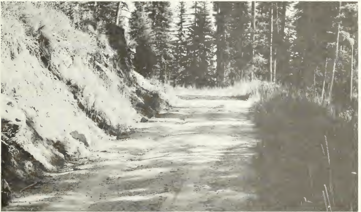
Figure 17.--Cut slope near maximum height of 6 feet (1.83 m)--structurally stable, but prone to sloughing. A cornice is beginning to build at the top of the cut.
