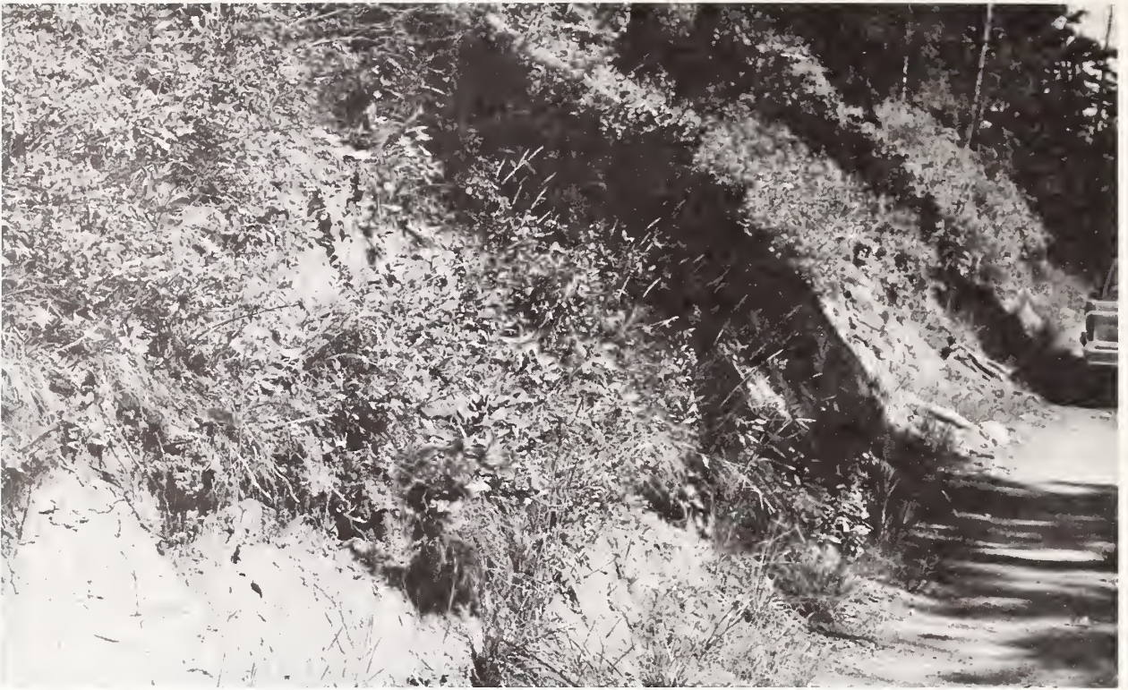
Figure 18.--Crack in a cut slope that is near the 6-foot (1.83-m) maximum height.
