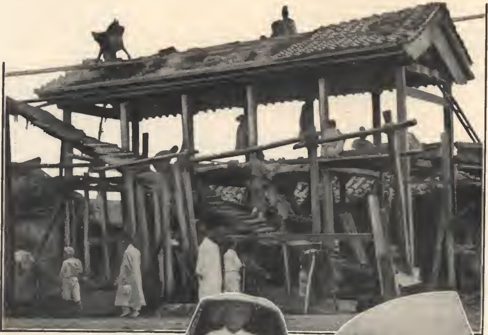
Korean methods of building—The roof is put on first of all, and the upper storeys are reached by a sloping gangway.
