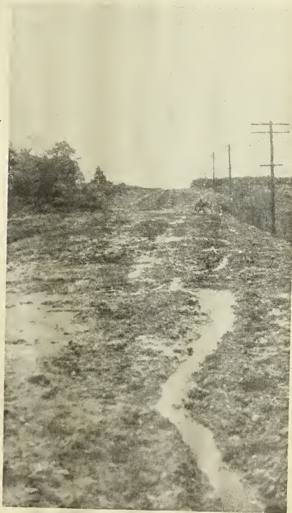
Fig. 4. - Overflow water may be trenched advantageously to other holes or cracks
