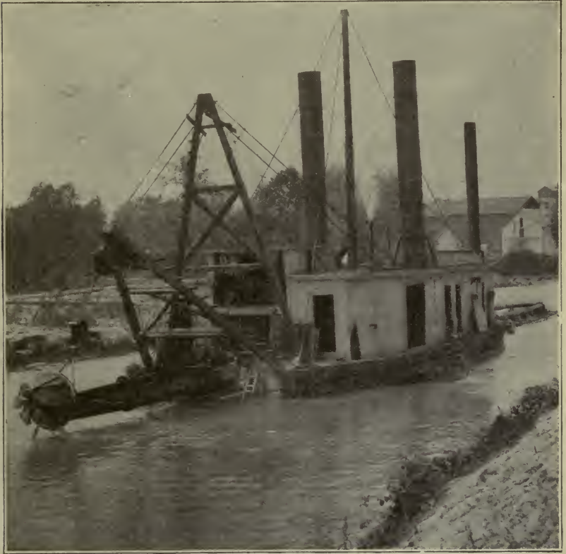
Fig. 61. Typical Hydraulic Dredge on Canal Construction Courtesy of Great Lakes Dredge and Dock Company, Chicago
