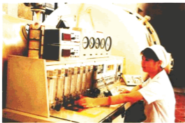
县医院高压氧舱 Hyperbaric Oxygen Cabin in Hui'an Hospital
