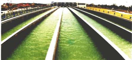
城南自来水厂 Chengnan Waterworks
