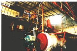
新型建材化工车间 Chemical Shop of New-style Building Materials
