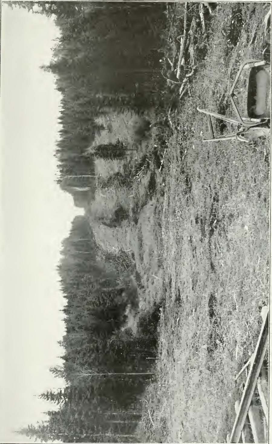
Cutting out a trunk road east from the town of Cochrane to the Abitibi River,
