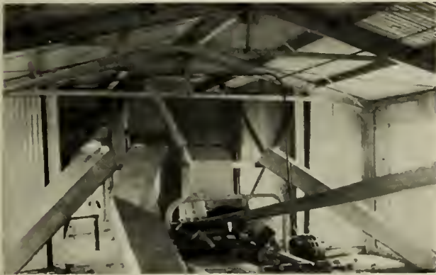
MOTOR AND MORSE DRIVE ON CONVEYOR
