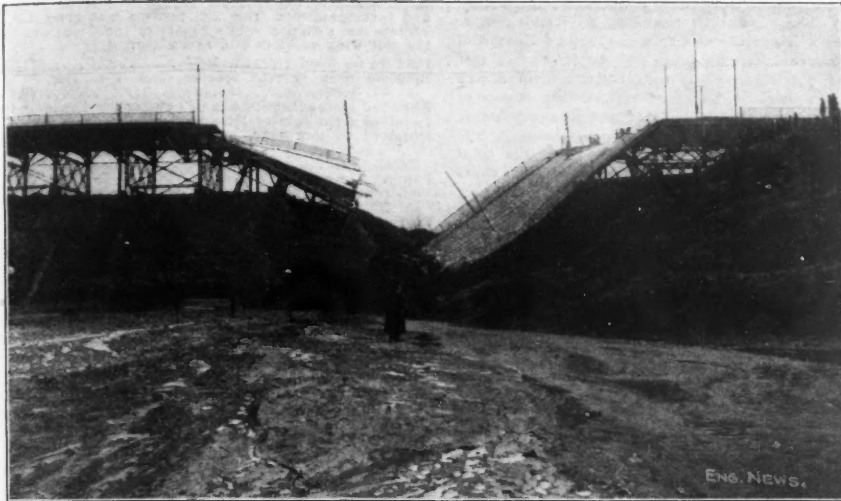
FIG. 3.—VIEW LOOKING EAST TOWARD WILSON AVE. BRIDGE, SHOWING EXTENT OF THE WRECK.
