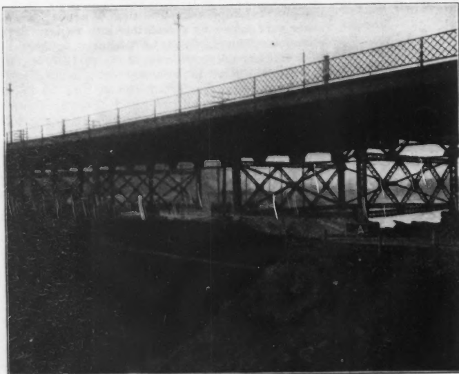
FIG. 2.—VIEW OF WILSON AVE. BRIDGE JUST PREVIOUS TO COLLAPSE, SHOWING EXTENT OF WASHOUT.
