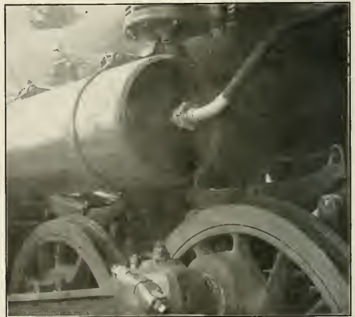
Main Reservoir Ball Joint Pipe Connection
