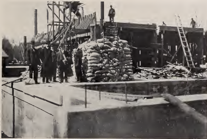
HODGMAN RUBBER CO. FACTORY, TUCKAHOE, N. Y. Test of floor shown on opposite page.
