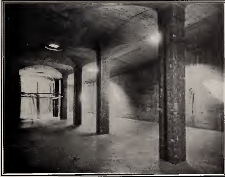
SLOW SAND FILTRATION PLANT, YONKERS N. Y. Interior of Clear Water Basin.
