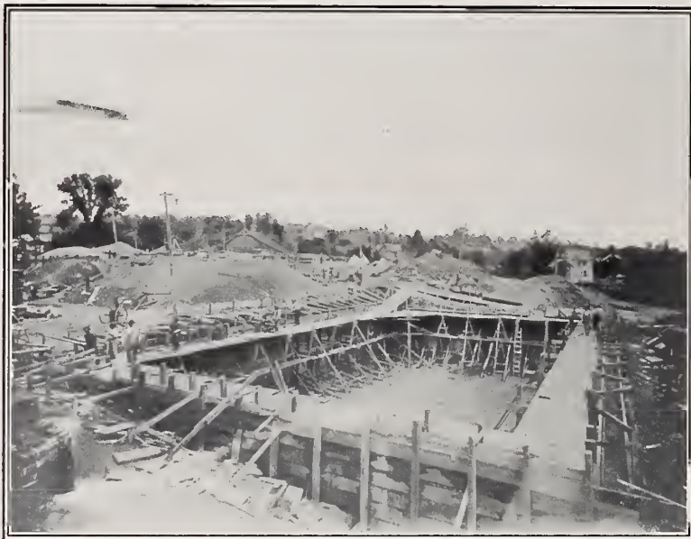
FILTRATION PLANT FOR ITHACA WATERWORKS CO., ITHACA, N. Y.
