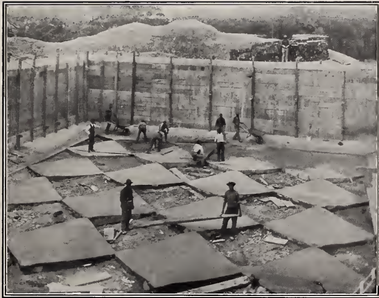
FILTRATION PLANT FOR ITHACA WATERWORKS CO., ITHACA, N. Y. Interior of Coagulating Basin, showing method of laying concrete in bottom.
