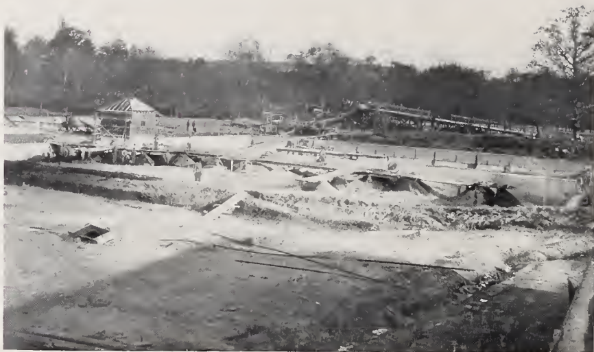
SLOW SAND FILTRATION PLANT, YONKERS N. Y.
