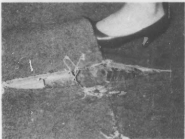
Torn or frayed rug should be repaired or replaced.
