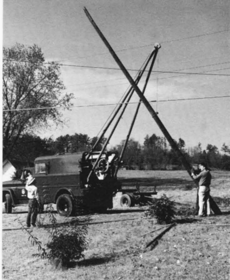
The Powell Telephone Co. follows the REA principle of area coverage and provides facilities where they are needed.
