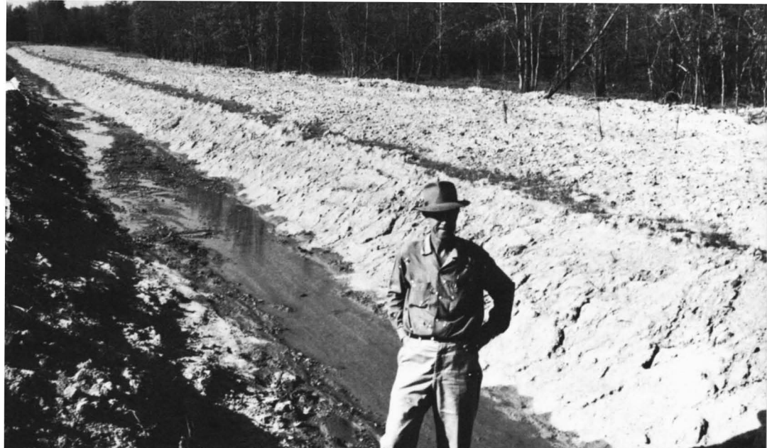
Soil Conservation Service technicians helped a farmer construct this drainage ditch in Logan County.
