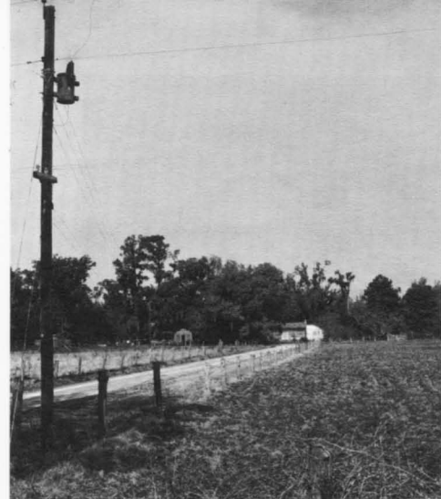
Typical REA-financed construction on the farm of T. L. Burgess in Clarendon County, S.C. The pole is used also by the telephone cooperative.
