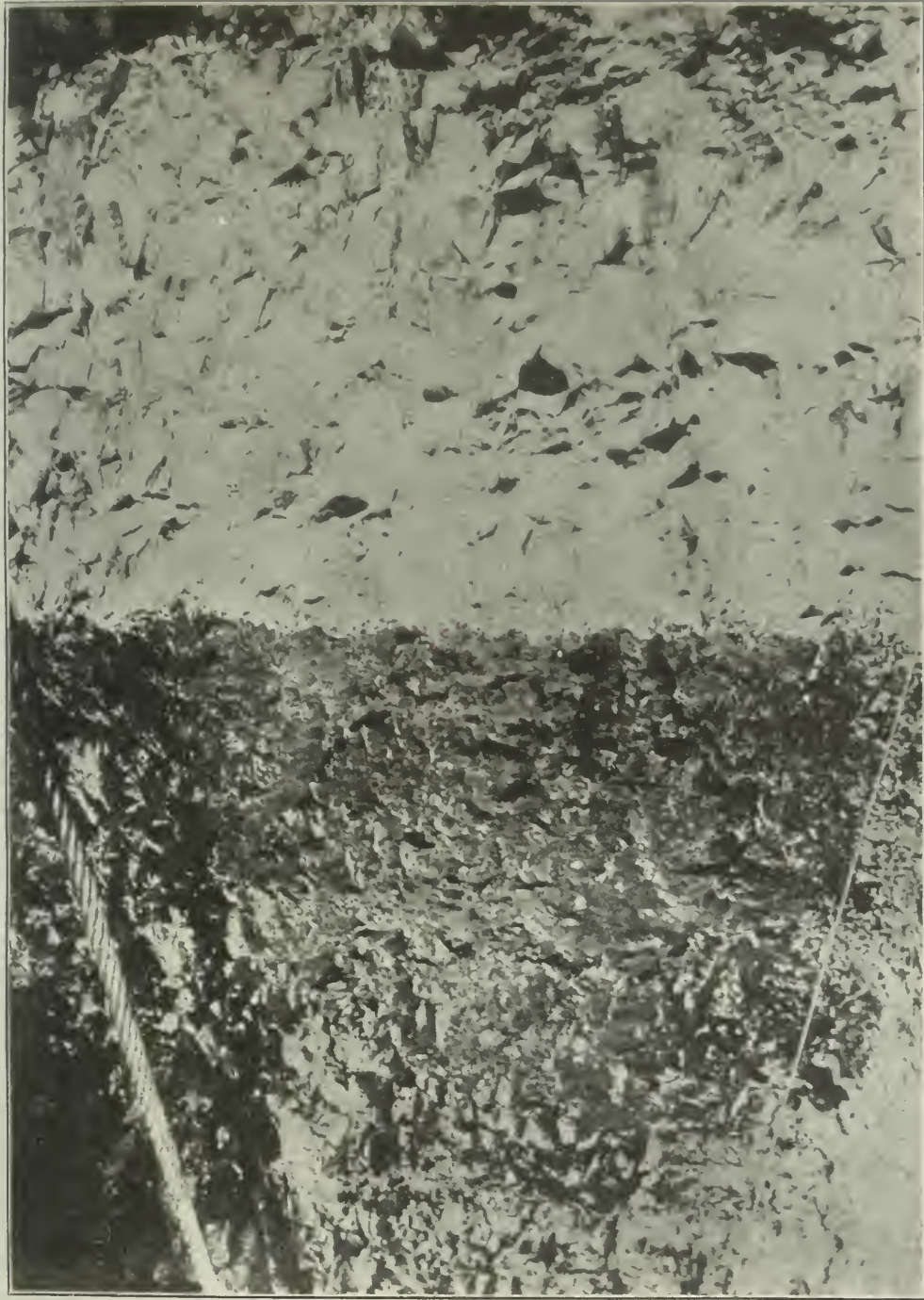
SIDE OF ROADWAY IN ALTOFTS MINE, SHOWING METHOD OF APPLYING STONE DUST AS A PREVENTIVE OF EXPLOSIONS.
