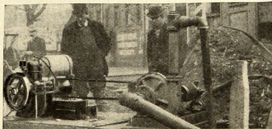
Gray Motor Pumping Water out of a Sewer at Norfolk, Va.
