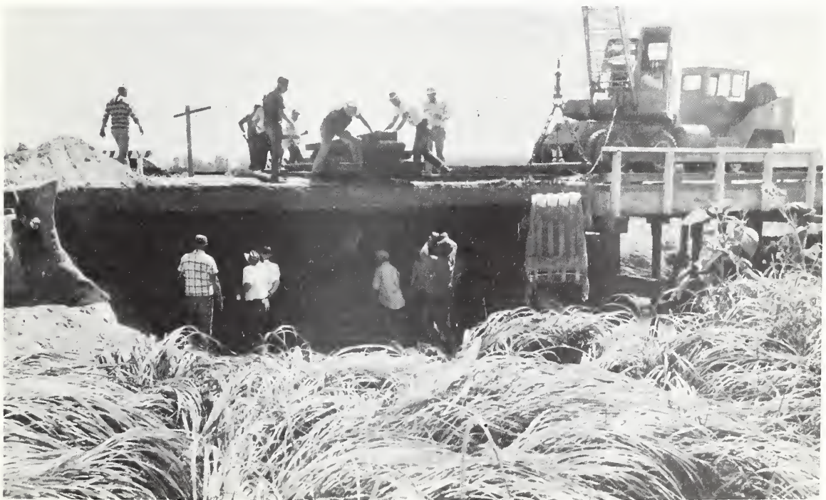
6. Storm runoff in August 1968 caused overflow adjacent to bridge on Highway 138 requiring extensive backfill to support concrete highway slab.
