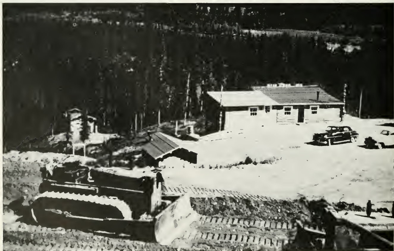
A highway bulldozer and the cars of some Bell System people are halted beside Bear Cub Inn, a typical lodge along the route
