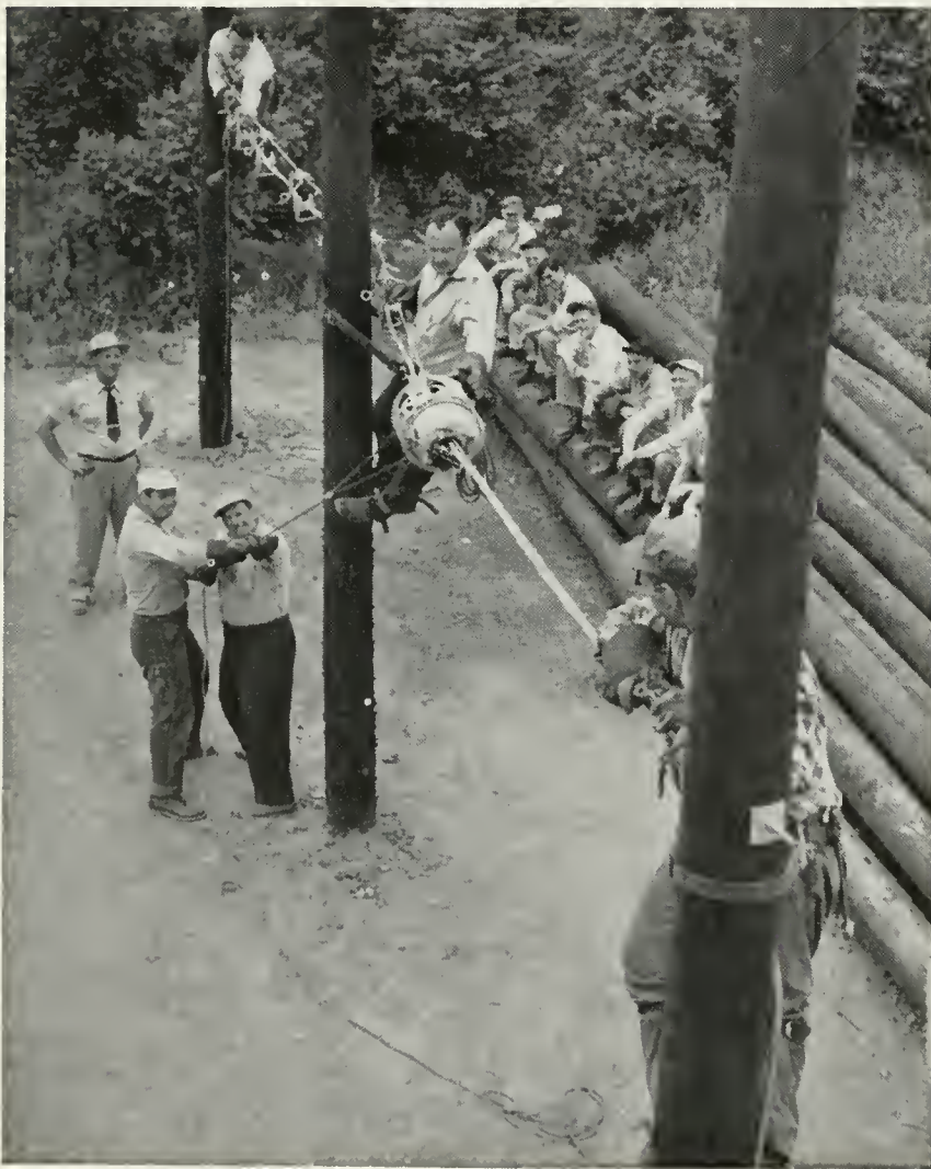
Necessary skill in the use of a cable lasher may be gained in plant school
