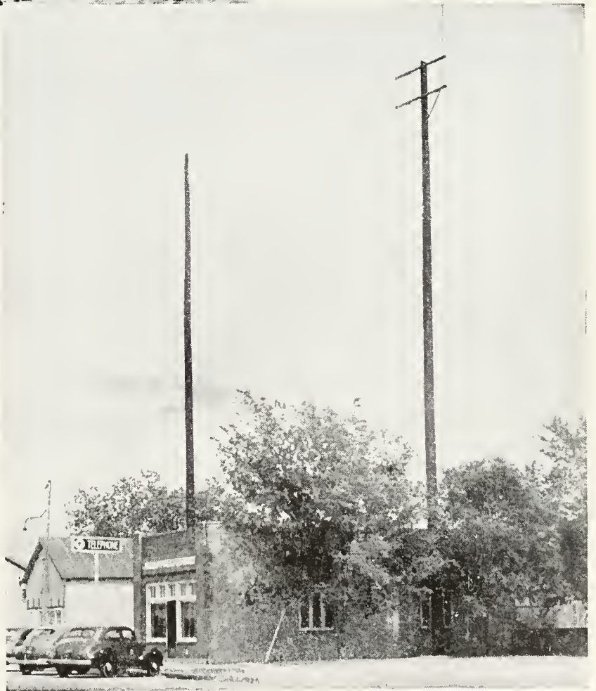
The telephone central office at Cheyenne Wells, Colorado, showing the antenna poles for the rural radiotelephone system. The transmitting antenna is at the left. The double antenna, at right, is for receiving
