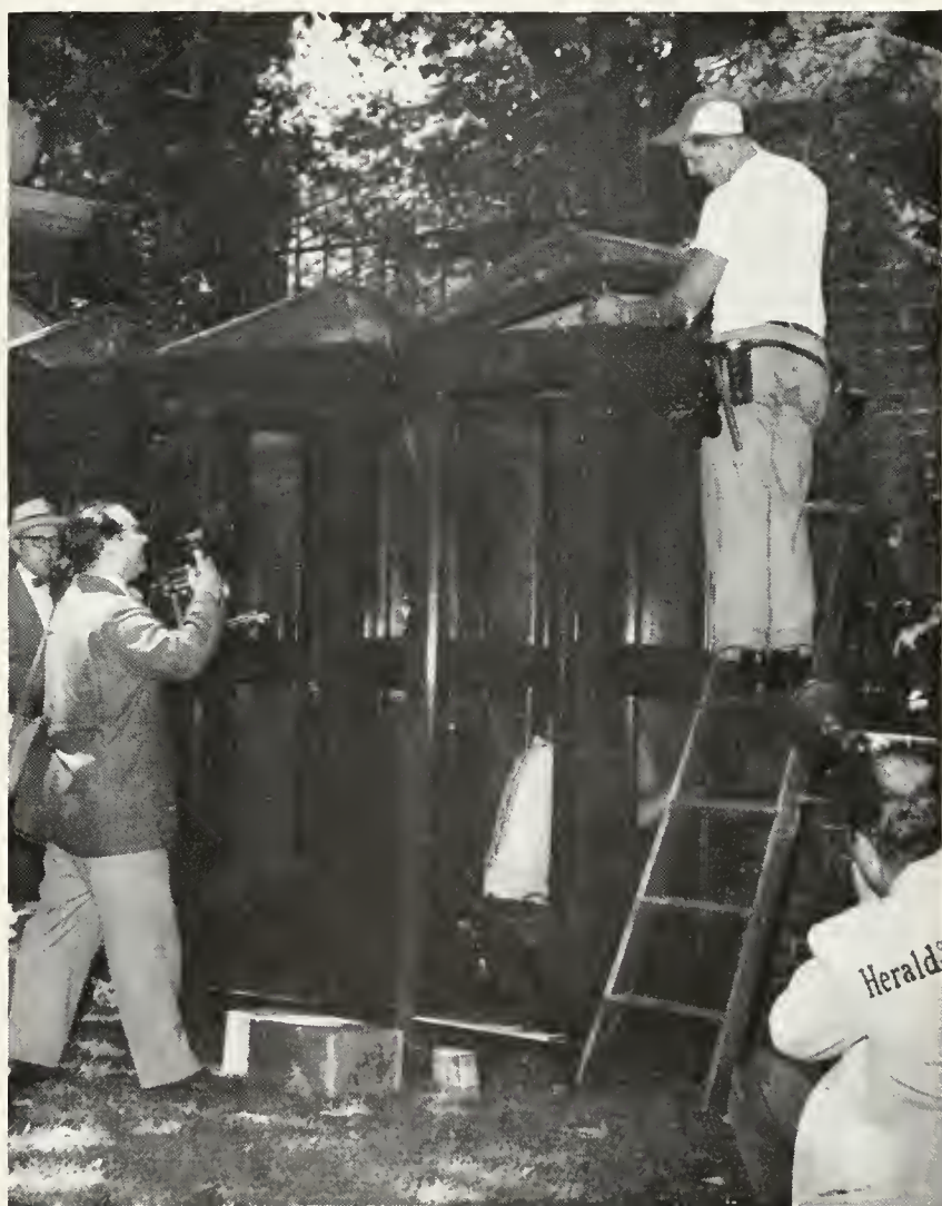
Swift installation of public telephones was good "news" to members of the press, radio and television keeping a 24-hour vigil at Astor Street. Telephone men had booths in operation an hour after they arrived
