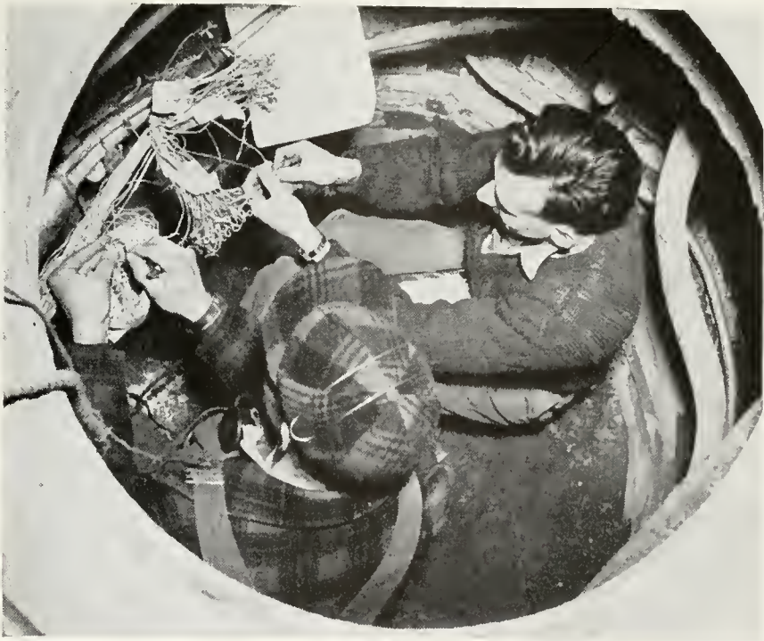
Cable splicers in a manhole cutting-in a new section of cable. Careful work and close coördination are required here not only to avoid interference but to match the circuits with absolute accuracy
