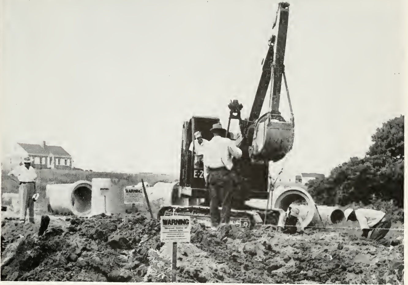
Warning markers have been placed along the cable route, and a telephone man stands by to assure that the digging is carried on without damage to the buried cable
