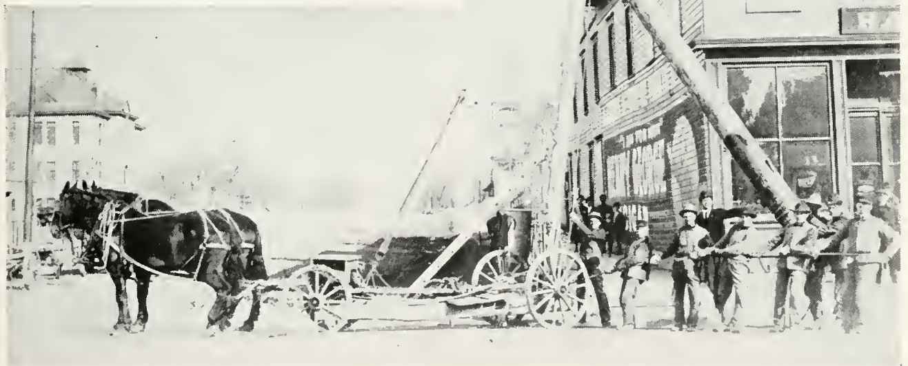
An "improved method" of pole raising, for which there probably was no "Practice"
