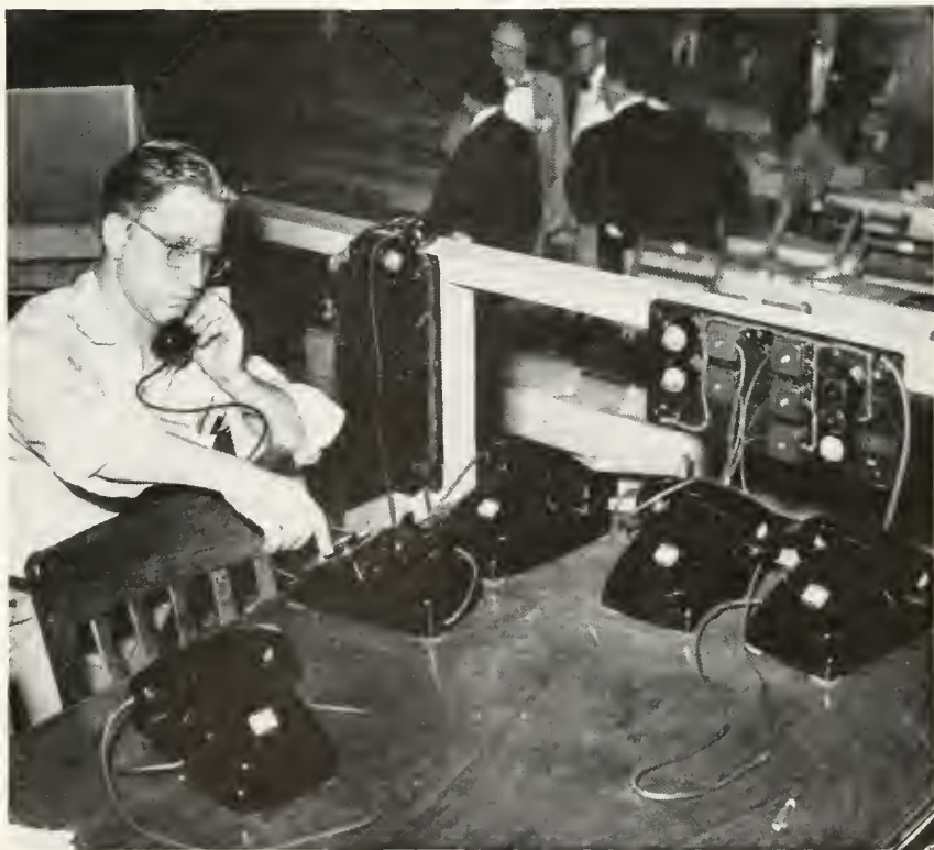
A plant man making one of the many telephone installations on the speaker's platform
