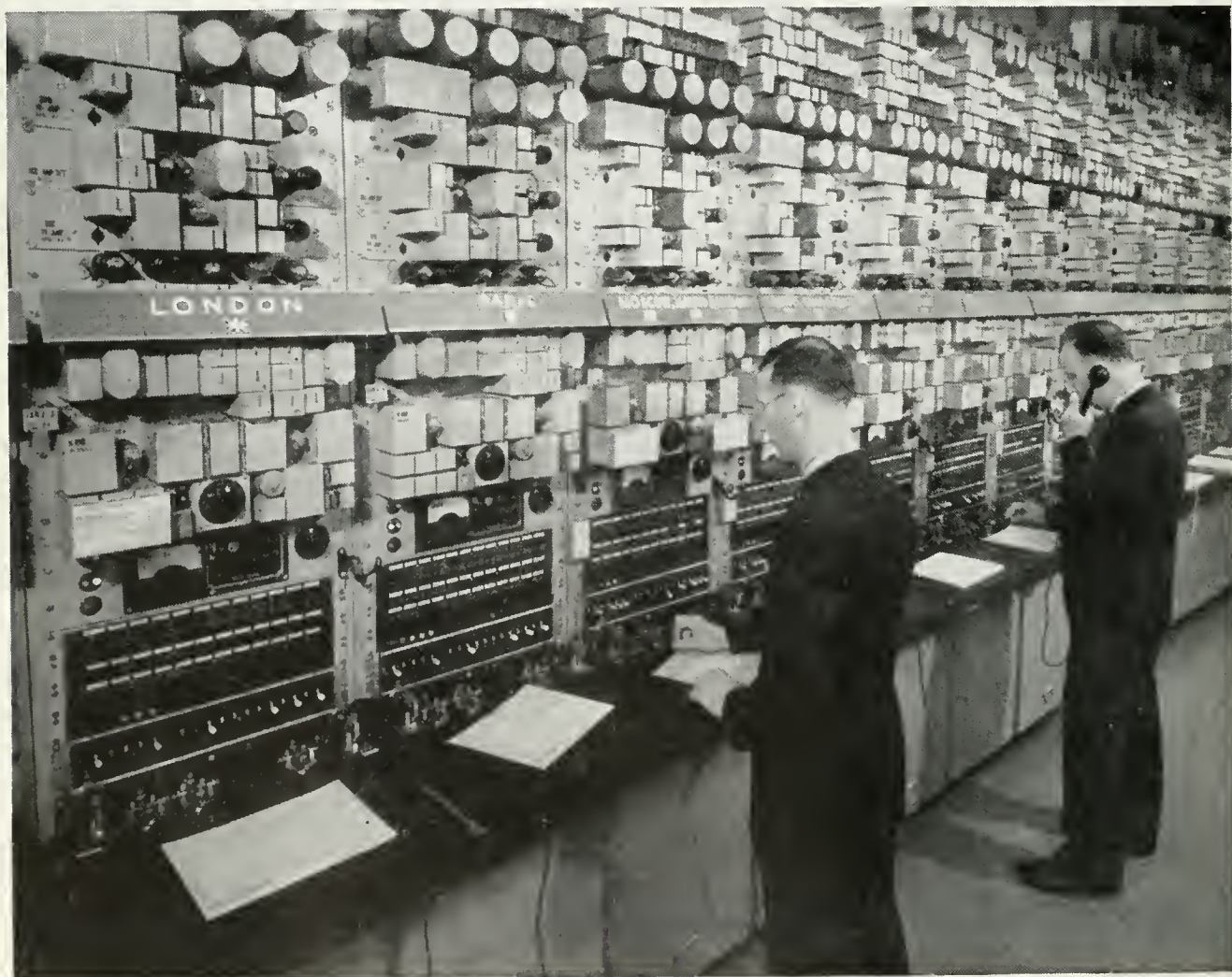
In the New York control room for overseas telephone service
