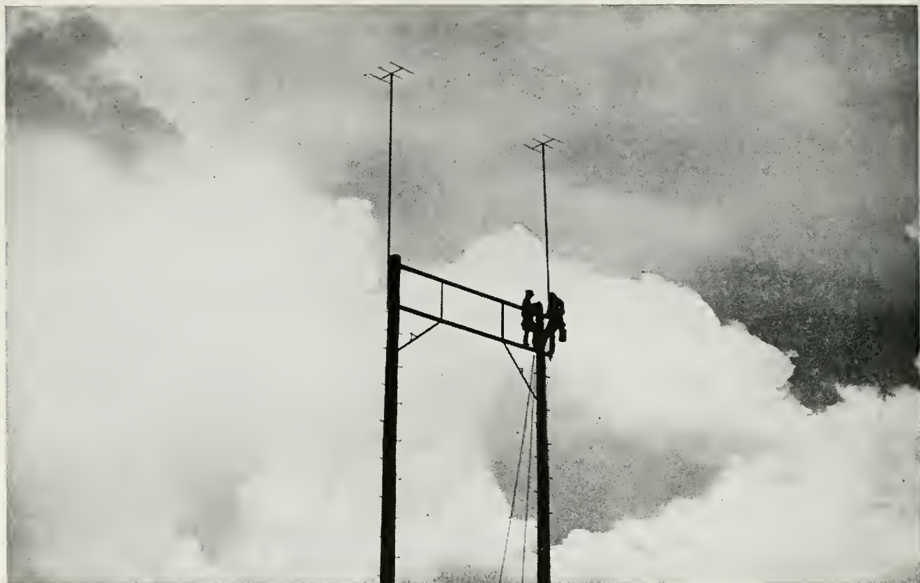
Erecting the antennas for the radiotelephone station at Anton, Colorado. This station provides two telephone circuits connecting with the Bell System wire circuits at Akron, Colorado, nearly 30 miles to the north
