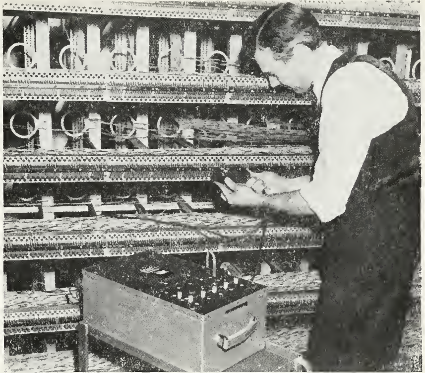
This outdated manual way of performing a line insulation test is being superseded by the automatic method shown on the opposite page
