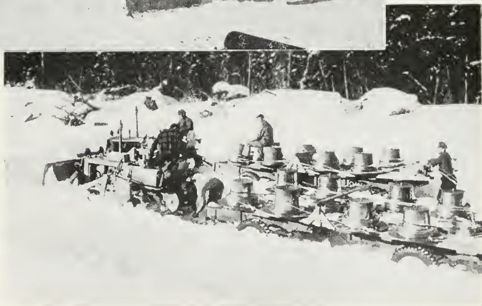
Above: A contractor's trucks at a supply dump. Right: Stringing wire proceeds despite the depth of snow
