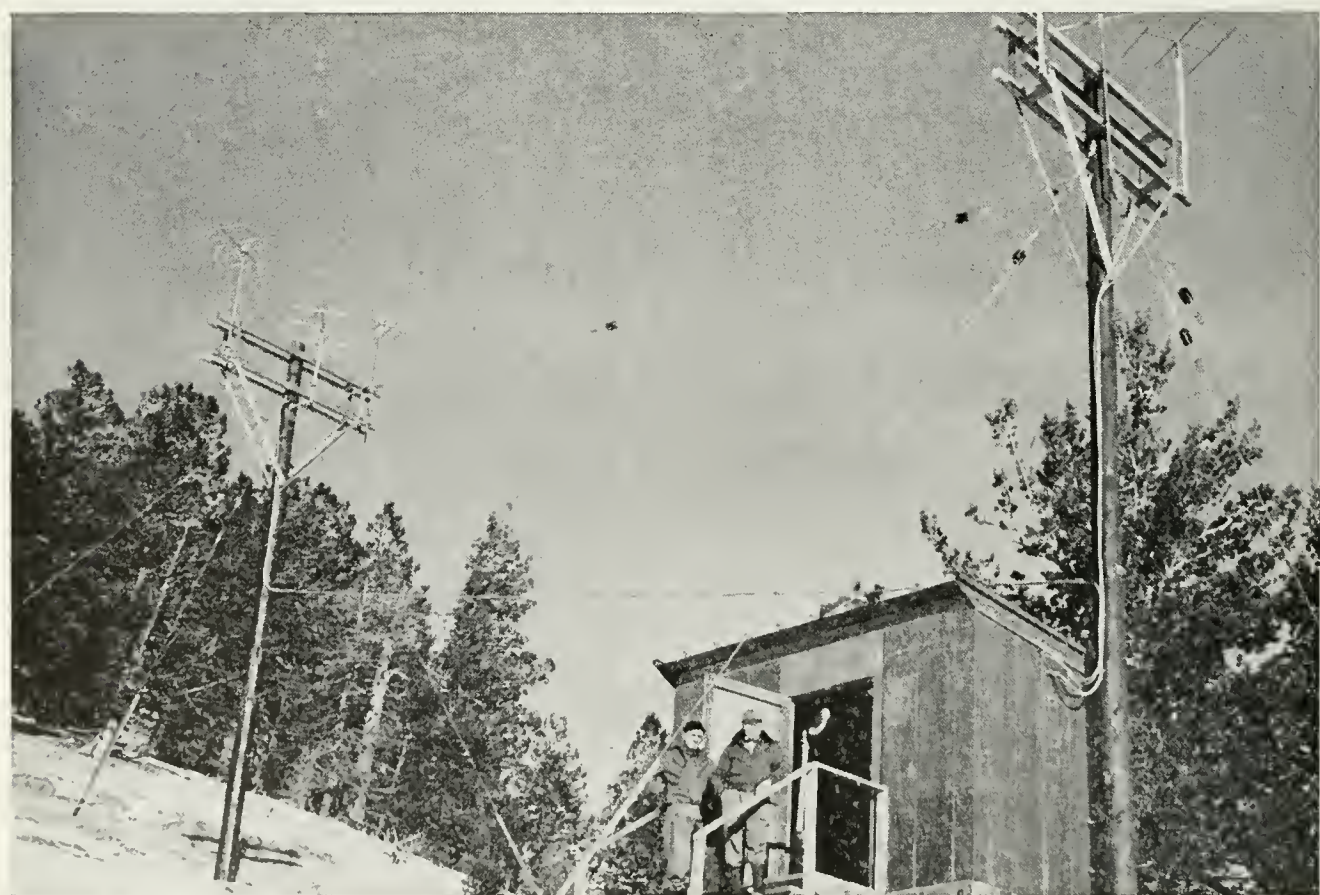
This radio repeater station on the 9300 foot summit of Escalante Mountain carries telephone messages to and from a new petroleum field in a remote section of Utah
