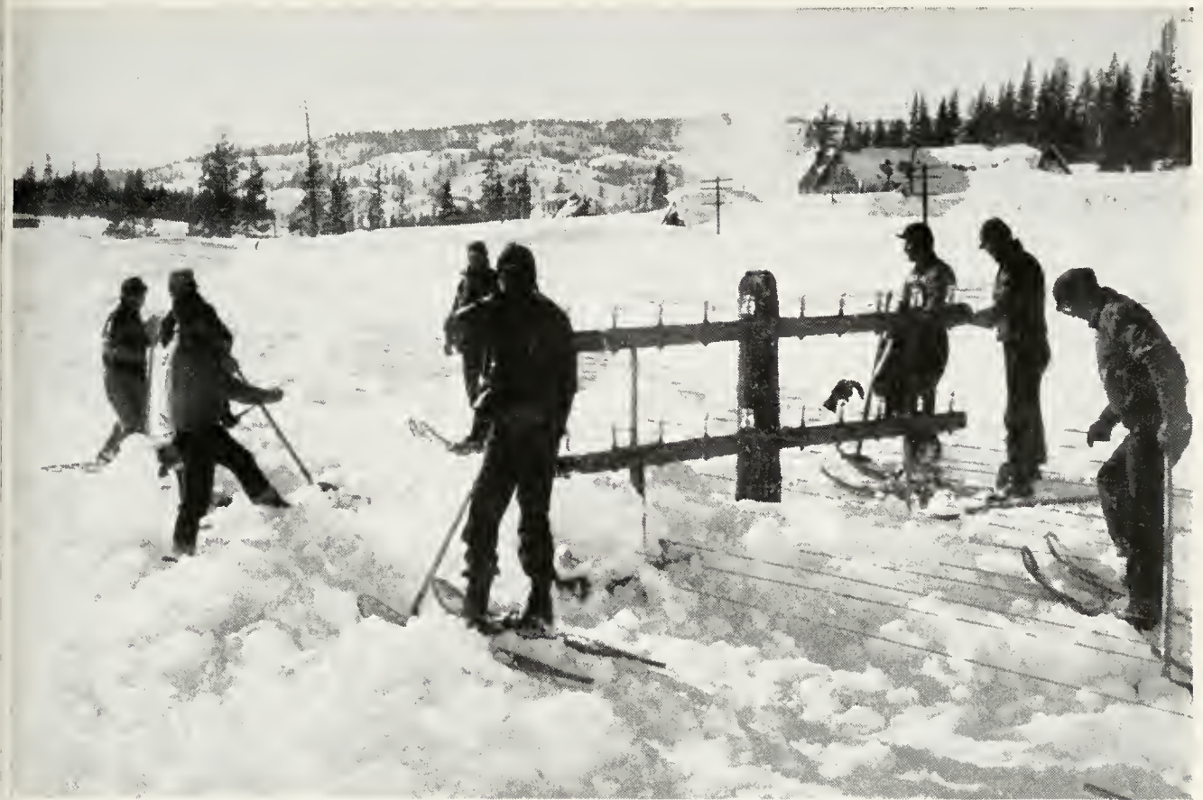
Digging down to telephone wires, to free them from their unaccustomed burden of snow, is an unusual form of preventive maintenance
