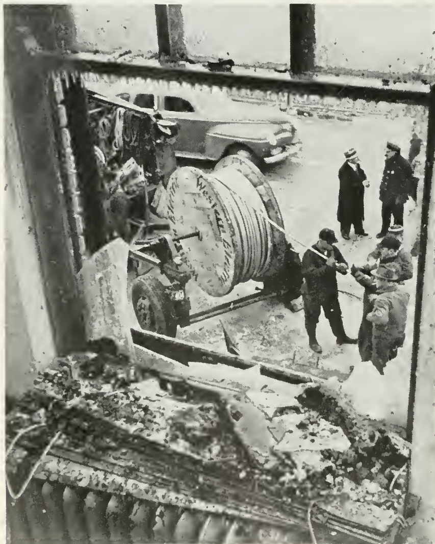
Service in the River Grove, Ill., central office was completely restored in eleven days after it had been gutted by fire—and without one personal injury
