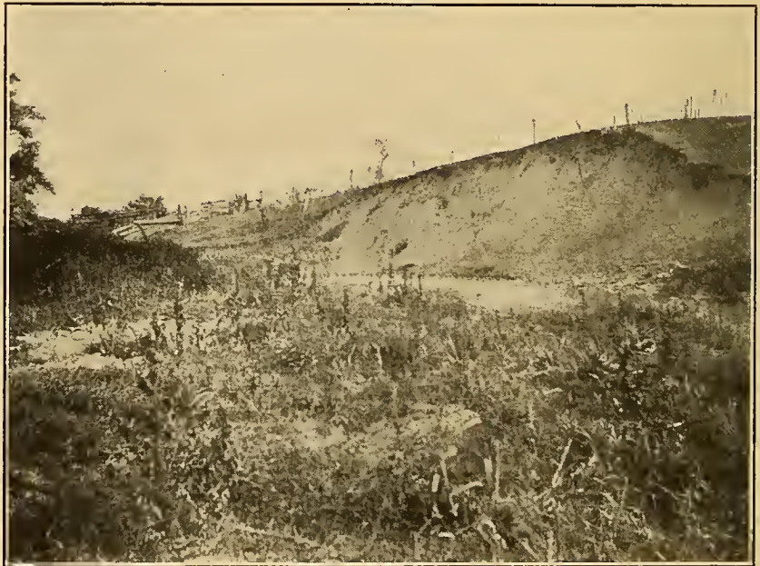
FIGURE 1.—Scour on the right Bank of the Lower Rouge.
