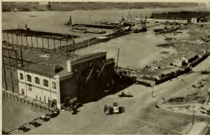
PIER 86, AND SITE OF NEW 1100-FOOT PIERS Cofferdam, mid center, being erected; undrained and un- excavated rock to right
