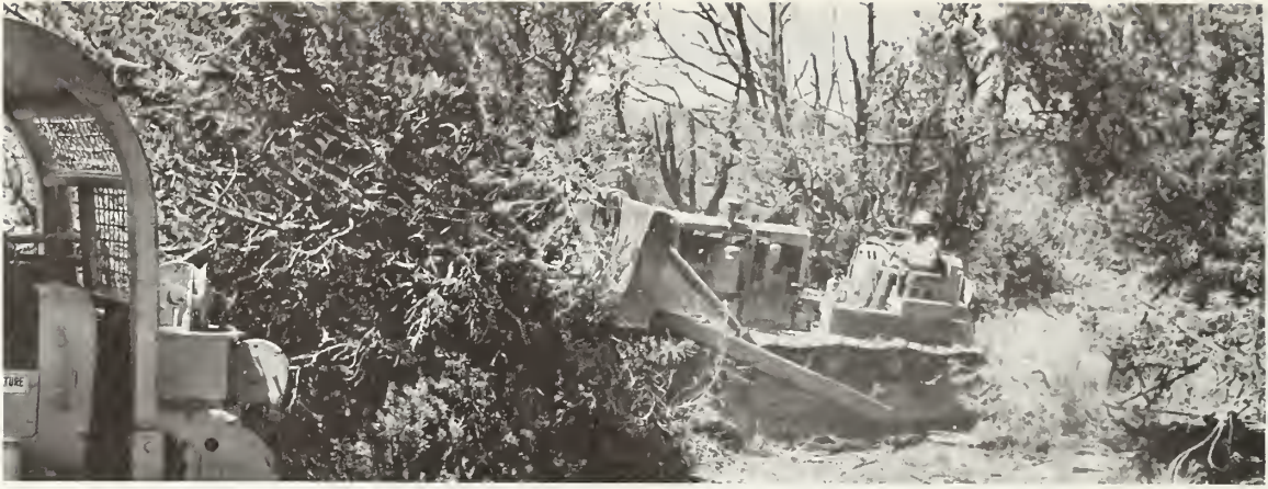
Bulldozing can be used either to destroy or to manage, pinyon-juniper woodland.
