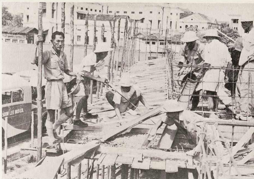
Placing concrete at first floor level for flats at Upper Hokien Street
