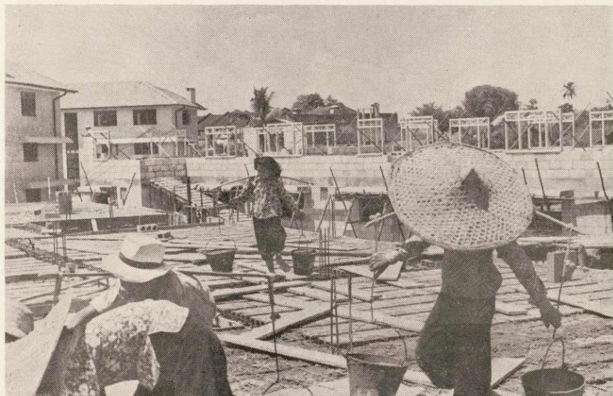
Part of nine blocks of workmen's flats at Delta Road in course of construction
