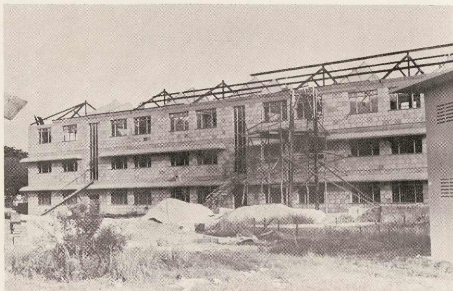
Part of eight blocks of workmen's flats at Kampong Java (Part III) nearing completion.
