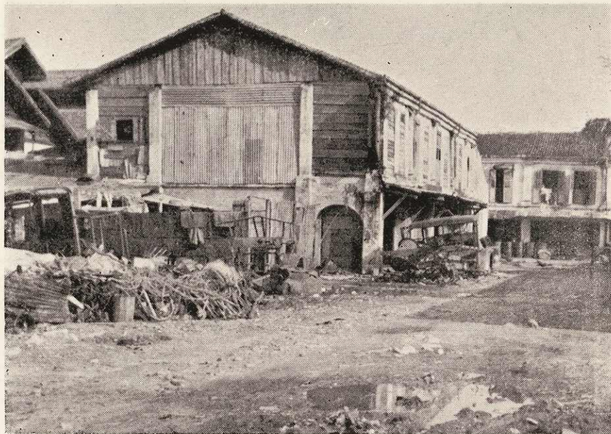
Dilapidated Shophouses. Covent Garden.
