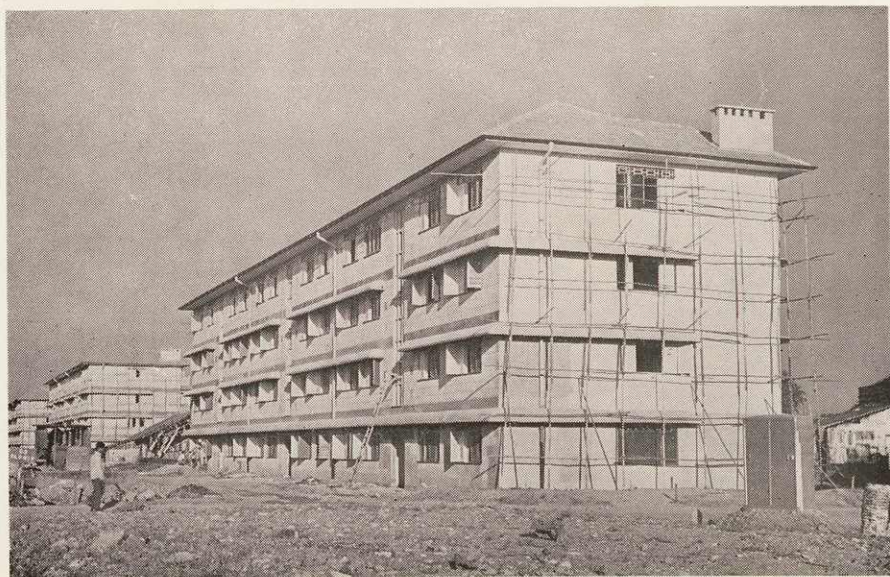
Some of the ten blocks of flats at Havelock Road nearing completion
