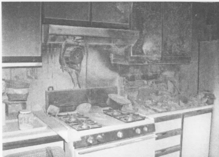
Left: Here are the results of a 2007 kitchen fire in the deputy chief of mission staff residence in Tunis, caused by an electrical short in a portable stereo situated next to the stove. Below: OBO engineer Dave Stobaugh says fire protection overseas depends on proven technology.
