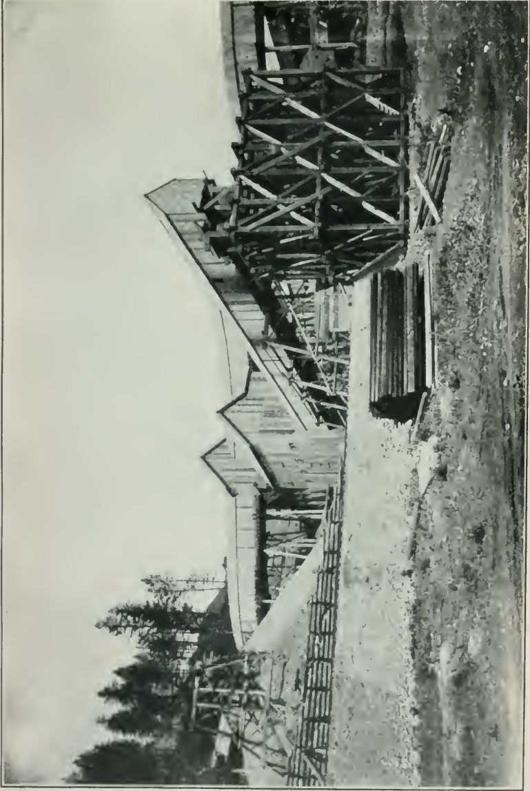
Fig. VII—Curlew Terminals. These handle the output from the Curlew, Gold Drop, and Monarch claims. At present the ore is delivered into cars from a travelling belt. Bins, however, will shortly be constructed.
