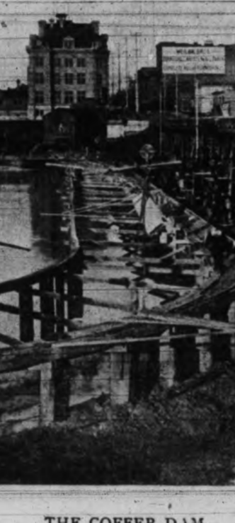
The picture shows the coffer dam, built to keep the water off the locality in which the work on the wall was progressing.
