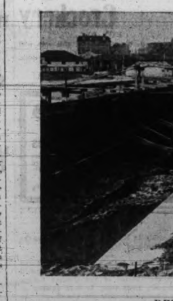
This cut shows the retaining wall in its early stage—about eight hundred piles driven deeply into the mud on the outside of the present bridge.
