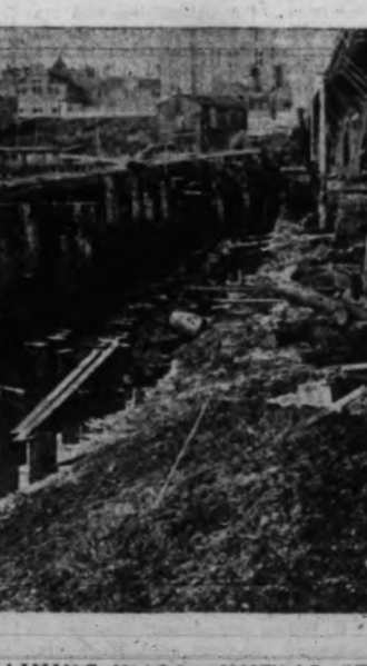
This cut shows the retaining wall in its early stage—about eight hundred piles driven deeply into the mud on the outside of the present bridge.
