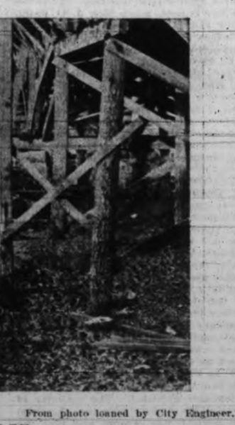
This cut shows the retaining wall in its early stage—about eight hundred piles driven deeply into the mud on the outside of the present bridge.
