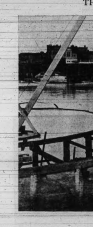
This picture shows the coffer dam, built to keep the water off the locality in which the work on the wall was progressing.
