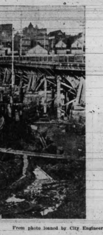
The picture shows the coffer dam, built to keep the water off the locality in which the work on the wall was progressing.
