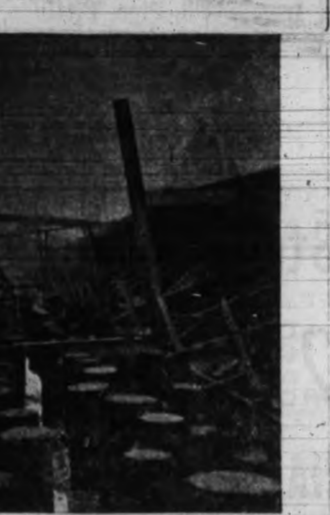
Photo loaned by City Engineer. RETAINING WALL. Showing how the piles are sawn off.
