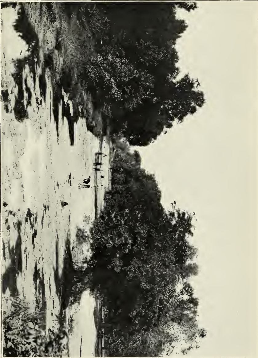
CREVASSE IN WARSAW-QUINCY LEVEE, WHERE THE EMBANKMENT HAS BEEN SWEEP OFF.
