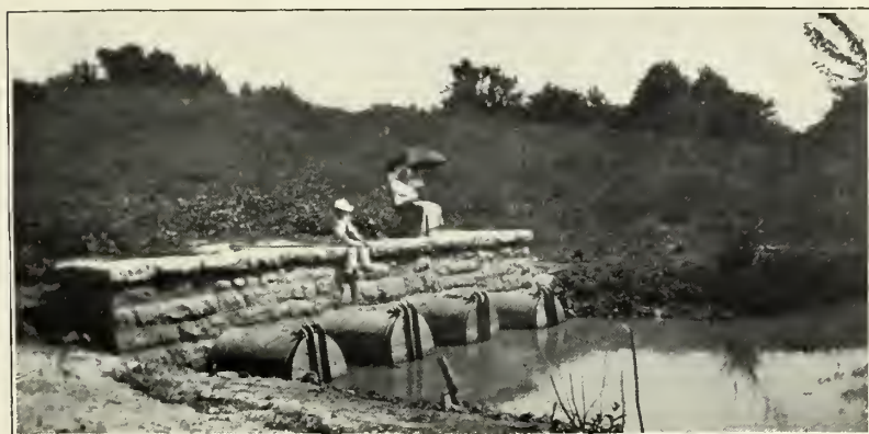
FIG. 2.—OUTLET END OF OUTFLOW CULVERT IN FLINT CREEK-IOWA RIVER LEVEE, SHOWING WOODEN VALVES.
