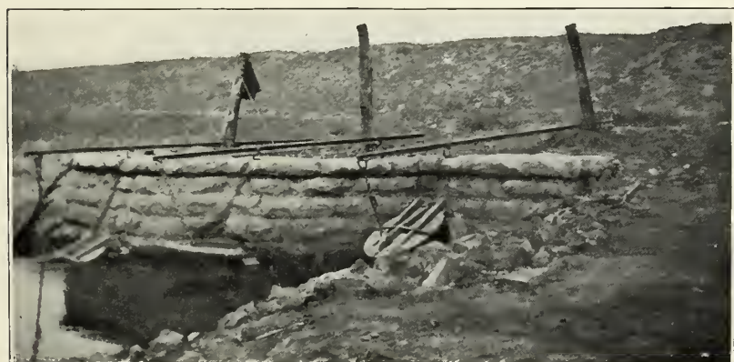
FIG. 3.—OUTLET END OF OUTFLOW CULVERT IN FLINT CREEK-IOWA RIVER LEVEE, SHOWING METHOD OF COUNTERBALANCING CAST-IRON VALVES.
