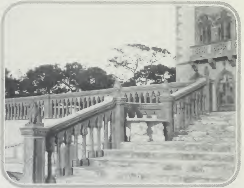
A detail of the steps leading down to the lower landing stage on the water front. These steps are twenty-five feet wide, of English veined marble, the balustrading being terra cotta, with the hand rail finished in brown glaze
