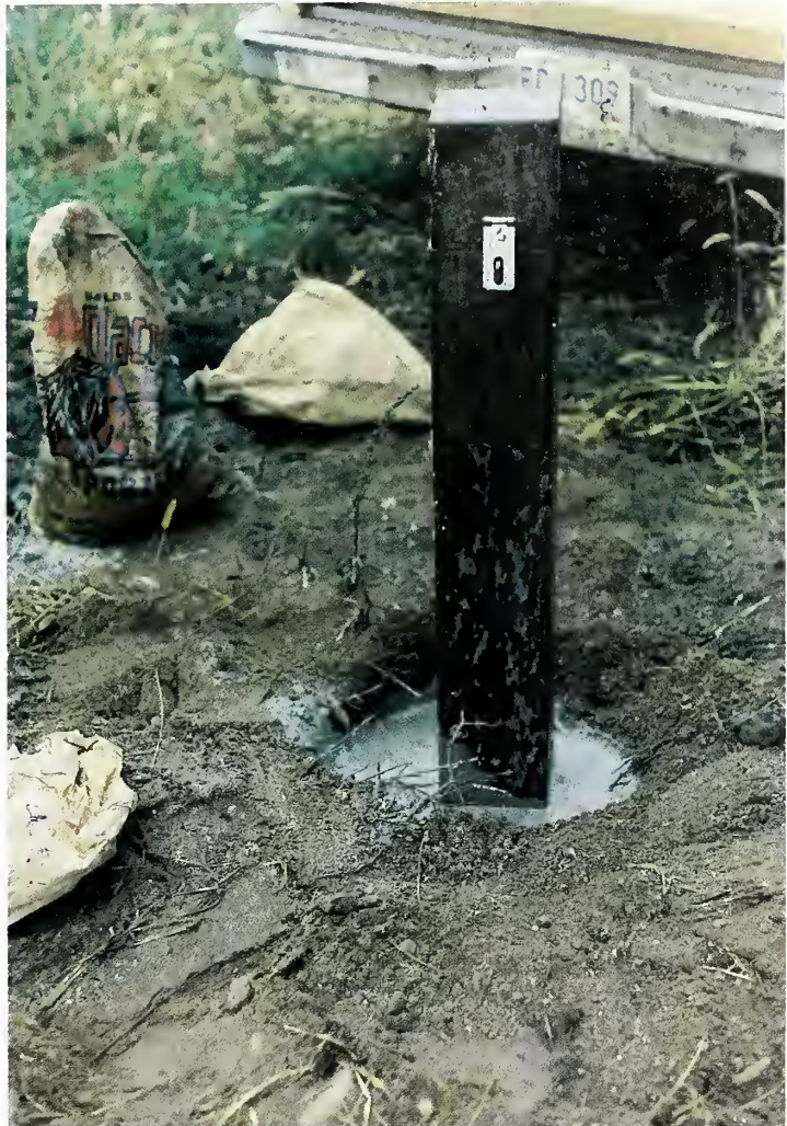
Figure 5. Metal, locked monitoring well protector.
