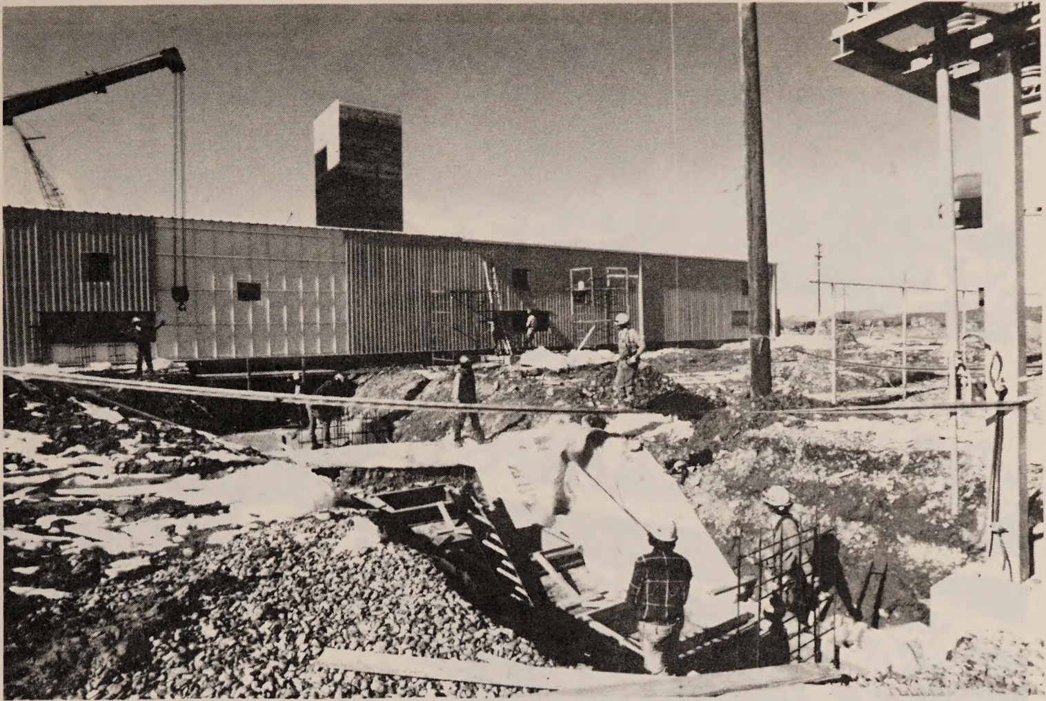
Figure 4-20. Excavation for the bus ducts from the switchyard to the power substation. (October 1981)
