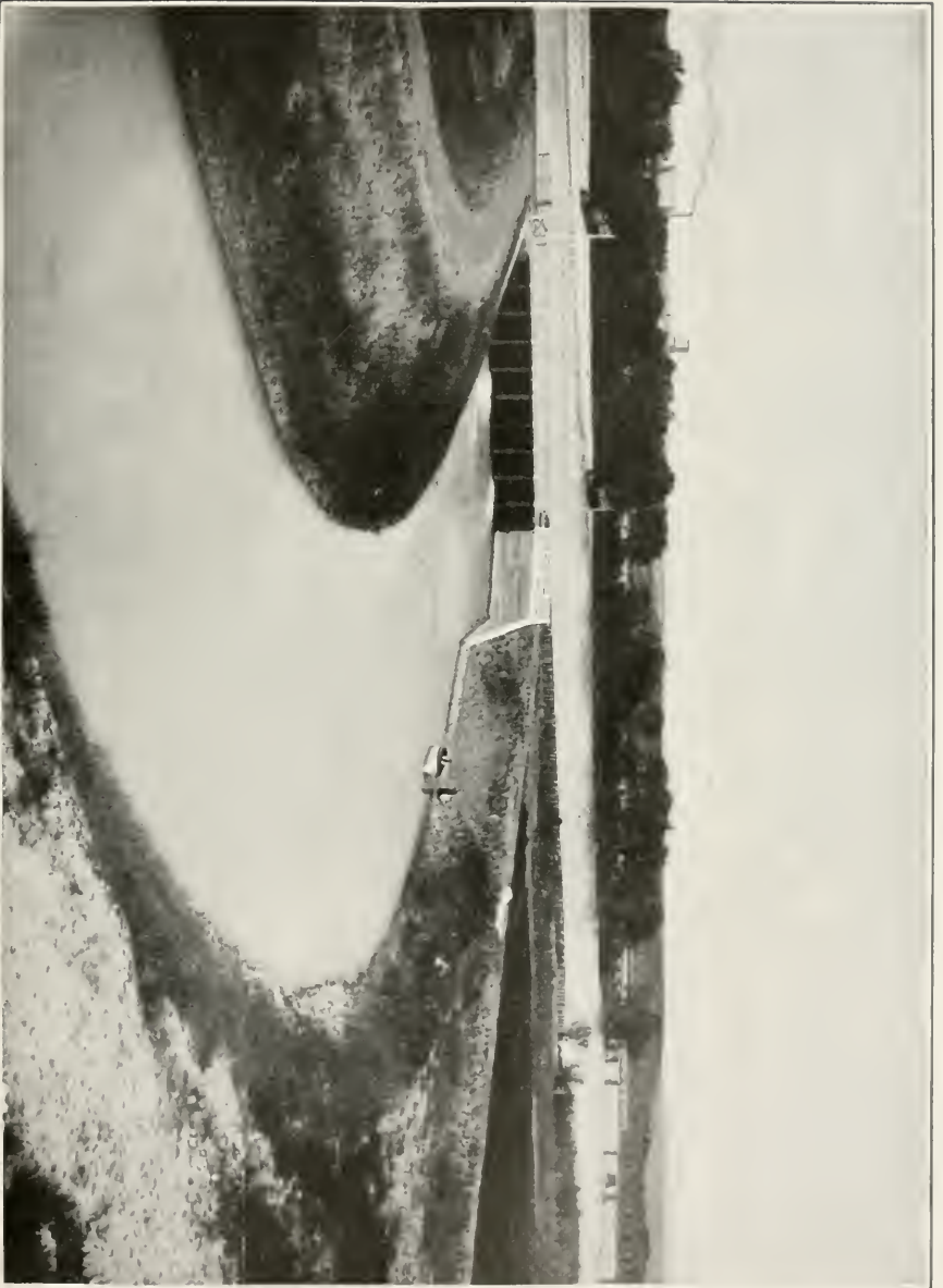
THE CALGARY SCHEME Headgate of the Main Canal of America's Biggest Irrigation Works, in the Canadian Northwest
