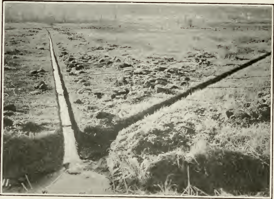
Not all of this work is in remote regions—Here are drainage ditches on Staten Island, New York—Constructed in connection with mosquito war, but incidentally the land grows paying crops of hay
