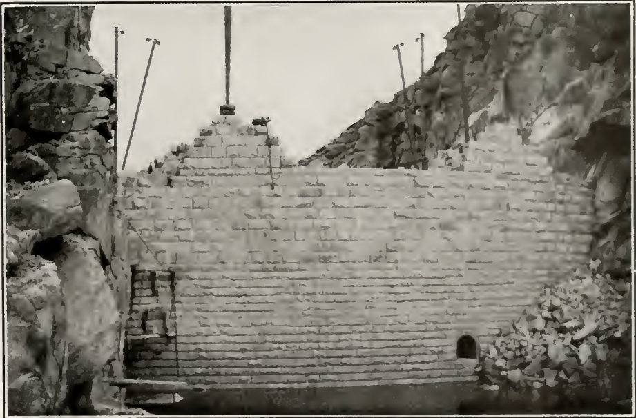
IRRIGATION IN THE NORTHWEST Upstream Face of the Great "Pathfinder" Dam, in Wyoming
