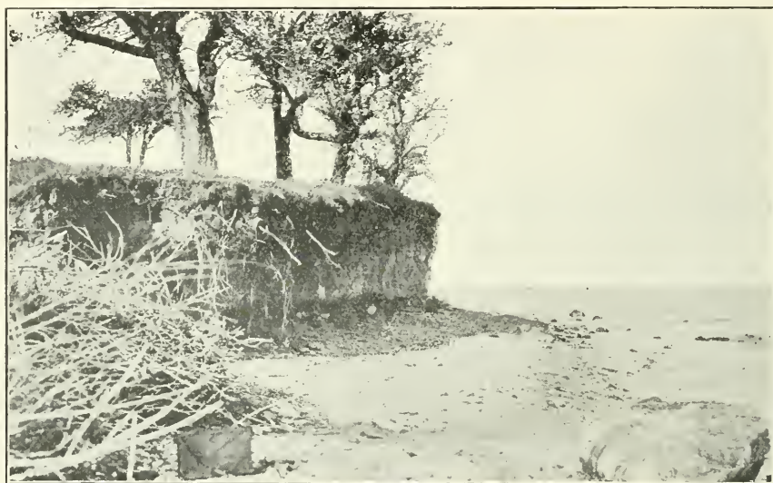
FIG. 6. Showing erosion of bank on Lake Ontario near the Government Fruit Farm at Jordan. Part of the apple orchard has been taken away in the last few years. Tree planting should remedy this breaking away.
