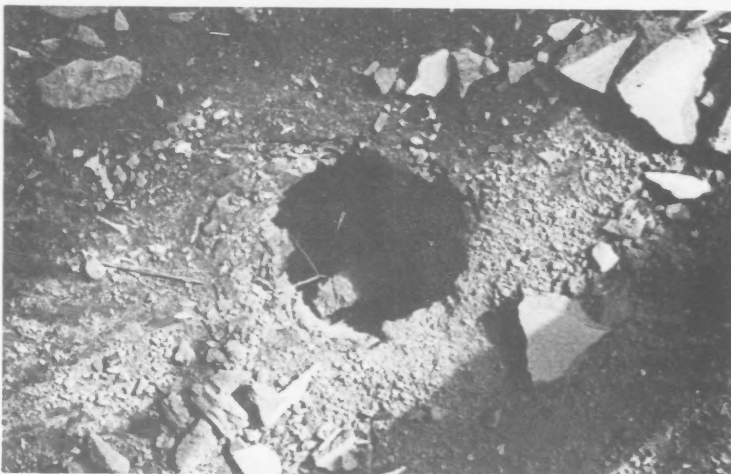
Seven-inch crater in stonemasonry floor outside embassy entrance marks impact of terrorist bomb. It blew out 115 large windows on front side of building.
