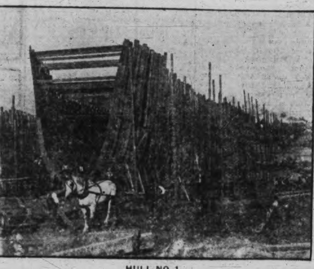
HULL NO. 1. The accompanying picture illustrates the rapid progress that has been made at the Cameron-Genoa shipyards in the construction of the first of the four ships to be built by this firm for the Munitions Board.
